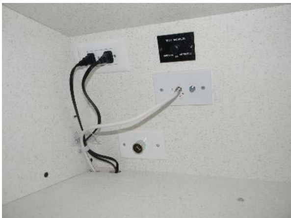
TV antenna switch
