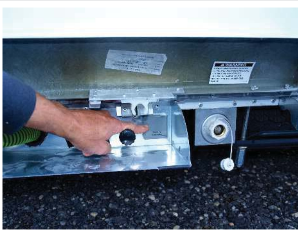
Cable TV connection location
