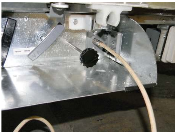
TV cable connected
