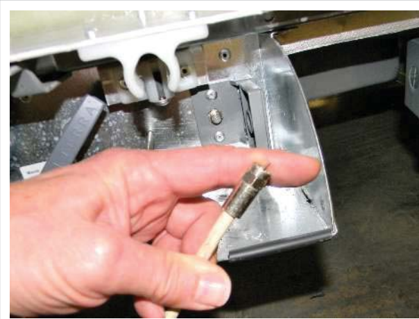
Coaxial TV connecting wire with screw-on end
