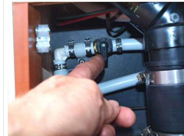
City water valve in closed, across-the-line position
