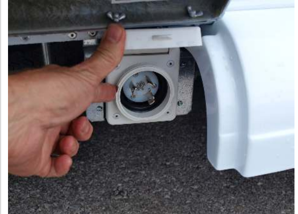
Shore power connection
