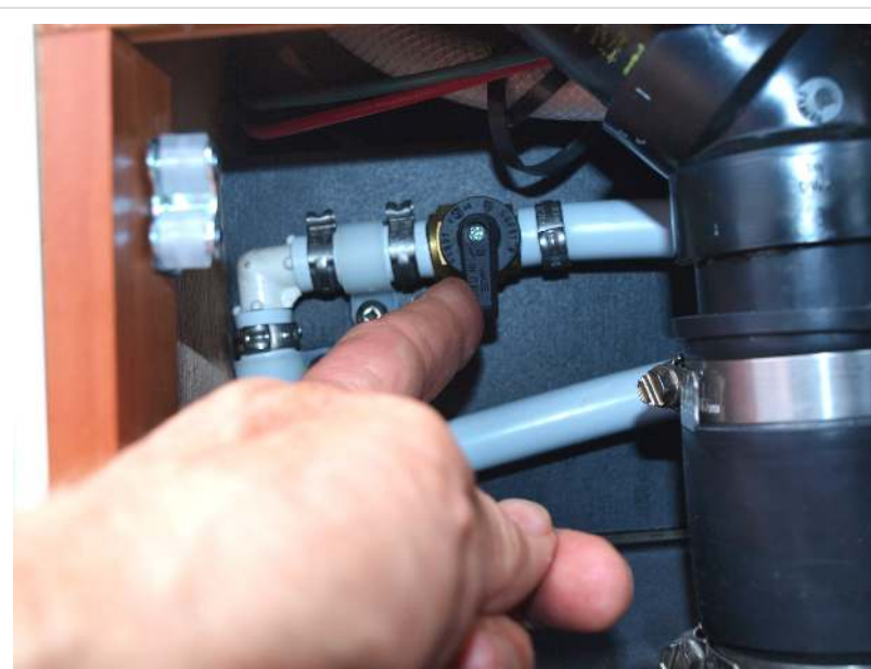
City water valve (shown closed)
