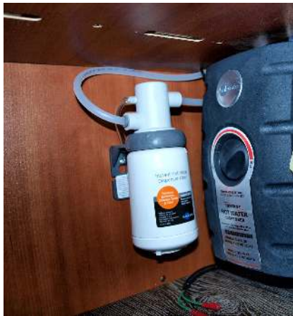
On-demand hot water system filter
