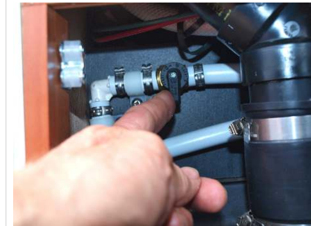
City water valve, shown closed
