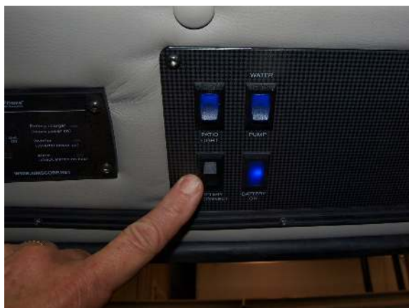
Battery disconnect switch
