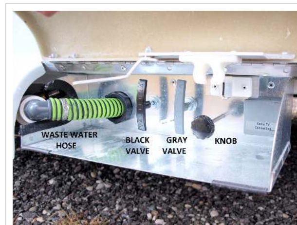
Waste water compartment controls
