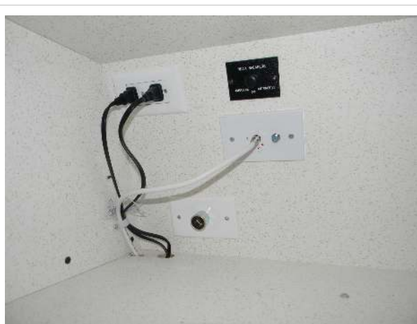
TV antenna switch
