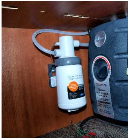
On-demand hot water system filter
