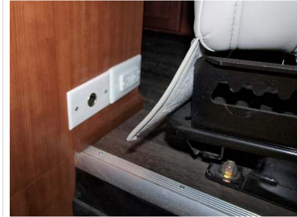
GFCI outlet behind rear captain's seat
