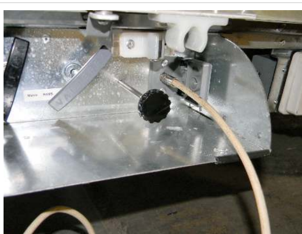
TV cable connected
