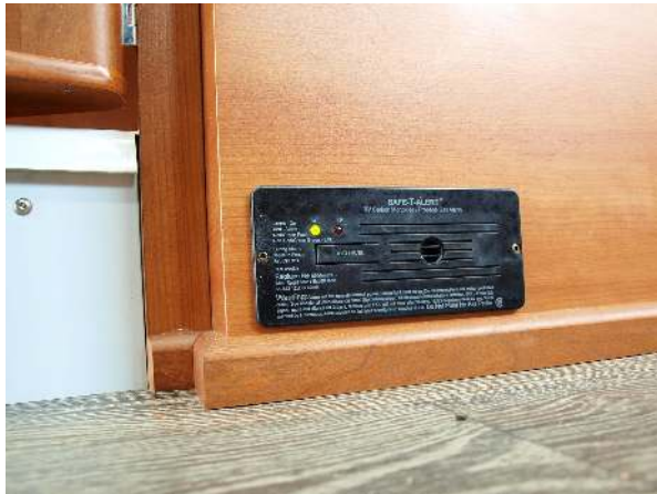
Propane and Carbon Monoxide alarm
