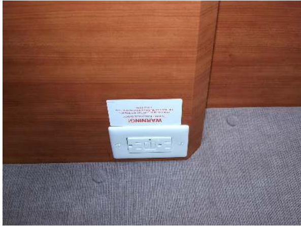
Galley GFCI outlet
