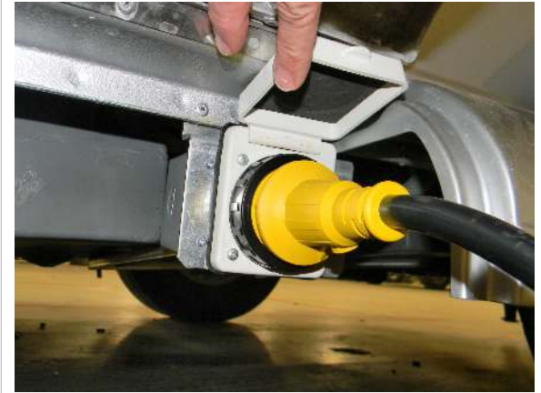
Attached shore power cord
