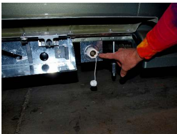
City water fill location
