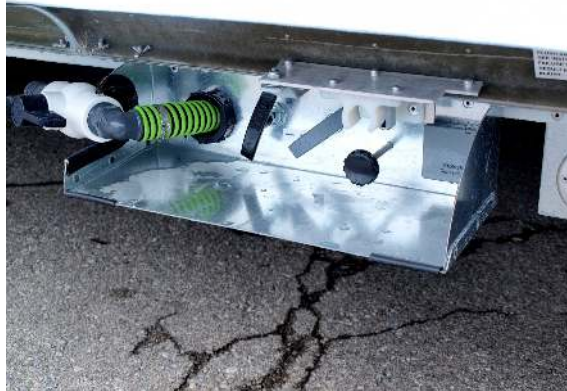
Waste disposal and cable TV access
