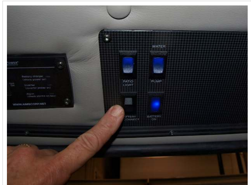
Battery disconnect switch
