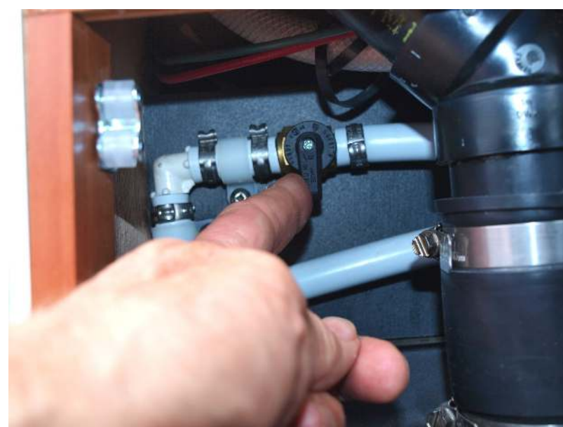
City water valve (shown closed)
