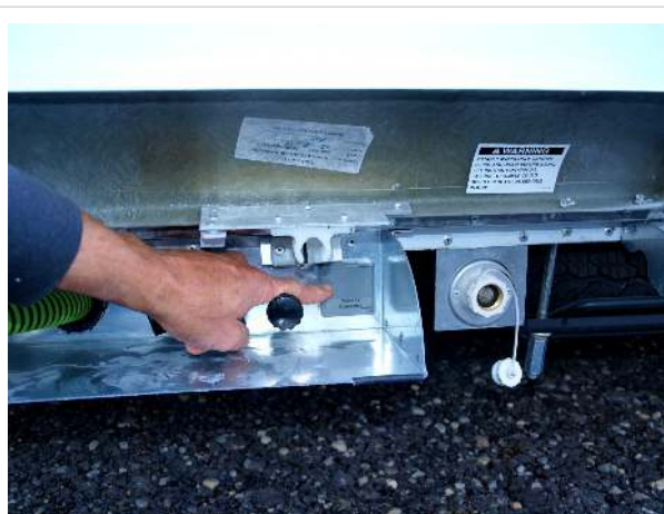
Cable TV connection location
