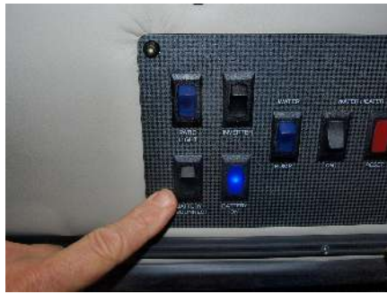
Battery disconnect switch
