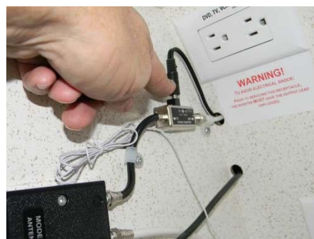
Antenna booster/power injector connection
