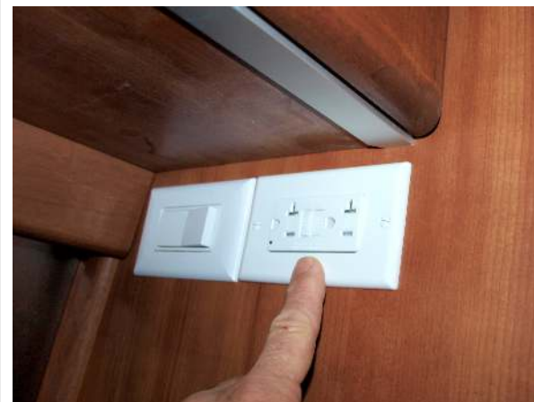
GFCI plug over galley
