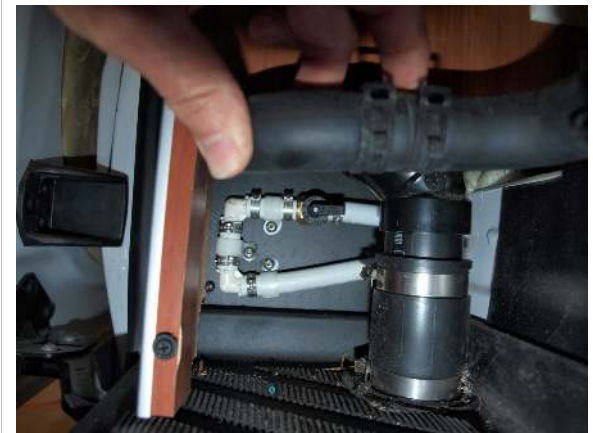
City water valve in open, along-the-line position
