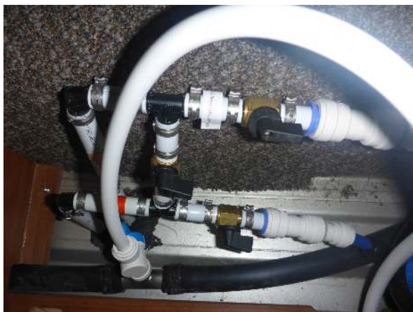
Bypass valves in normal position - all black handles point toward the front of the Roadtrek
