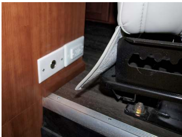
GFCI plug behind rear captain's seat
