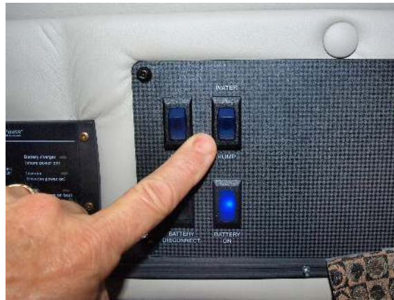
Water pump switch location with big inverter
