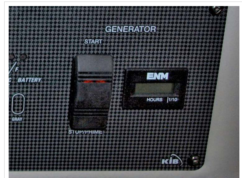
Propane generator control
