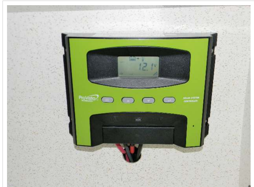
Solar controller in cabinet above galley
