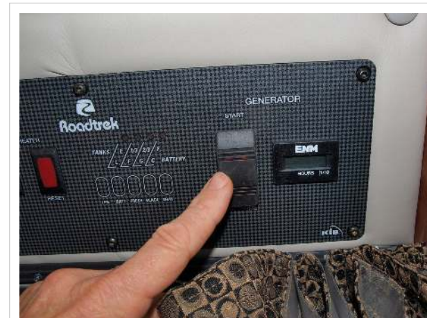
Generator switch and hour meter
