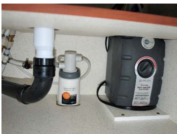
On-demand hot water system filter
