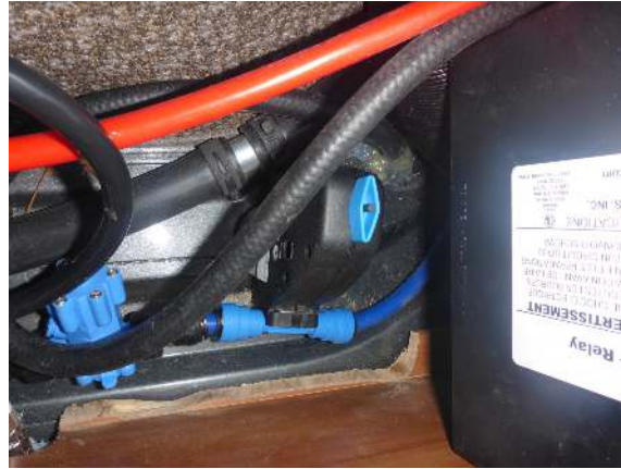
Frost control valve in tripped position
