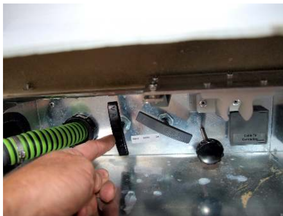
Waste disposal and cable TV access
