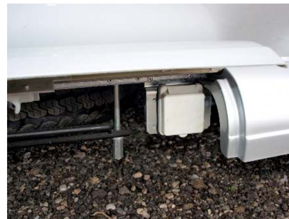
Shore power connection
