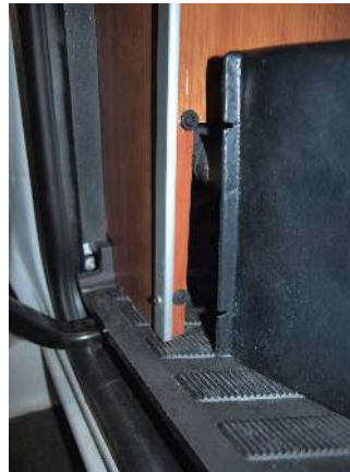
Screws holding plastic radiator cover on
