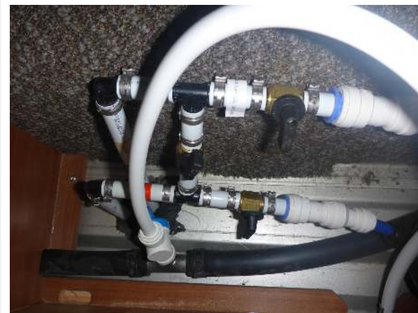
Valves turned to bypass position - all black handles pointing down or up
