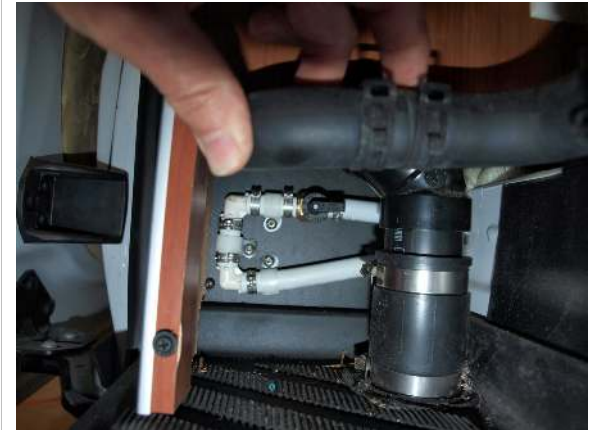
City water valve in open, along-the-line position
