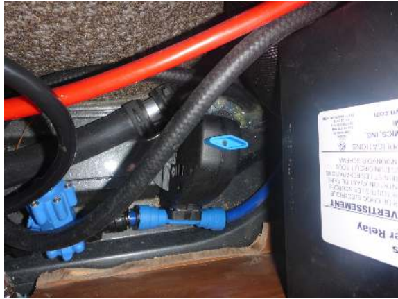
Alde frost control valve in operating position
