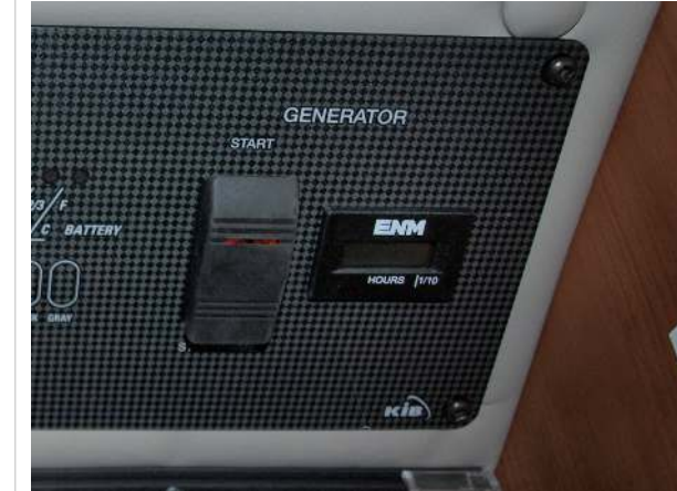
Generator switch and hour meter
