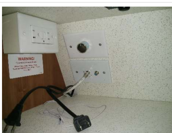
TV antenna and cable connections
