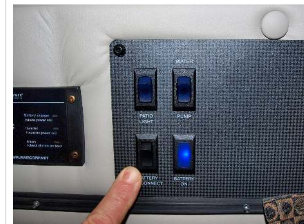
Battery disconnect switch
