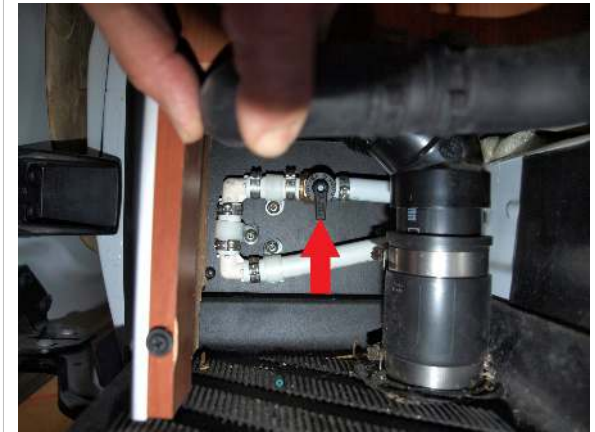
City water valve in closed, across-the-line position
