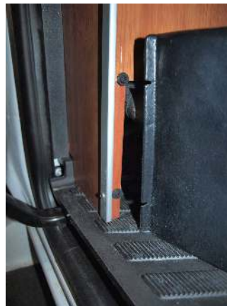
Screws holding plastic radiator cover on
