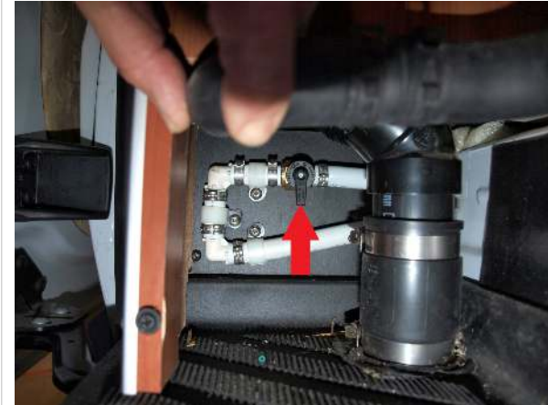
City water valve (red arrow) in closed position - handle across line
