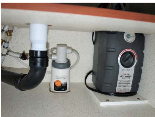
On-demand hot water system filter
