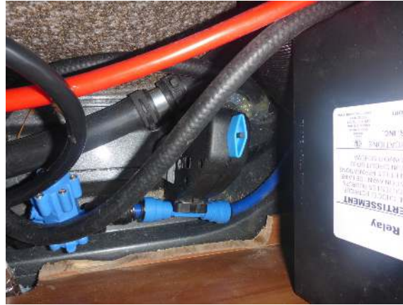
Frost control valve in tripped position
