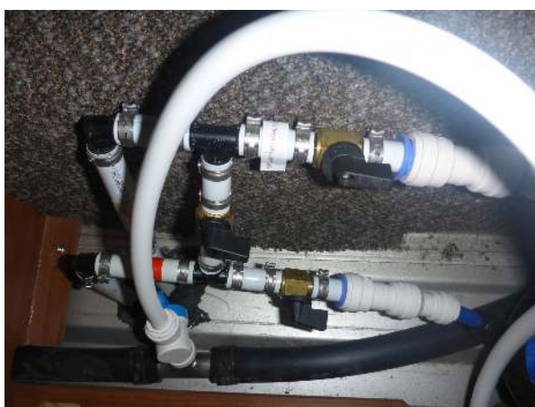
Bypass valves in normal position - all black handles horizontal
