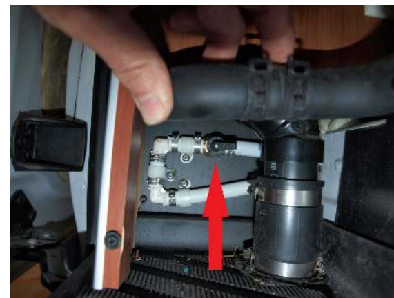
City water valve in open, along-the-line position
