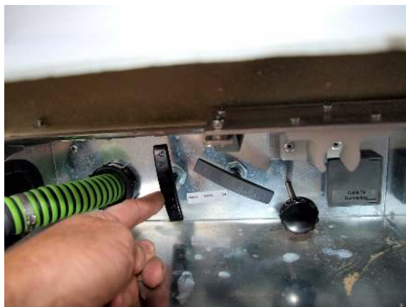
Waste disposal and cable TV access
