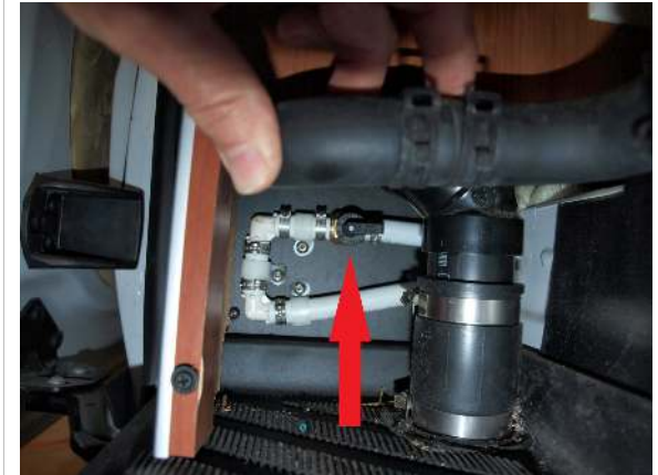
City water valve in open, along-the-line position
