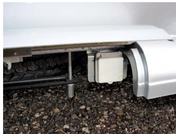
Shore power connection
