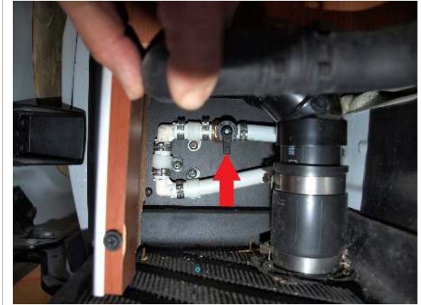
City water valve in closed, across-the-line position
