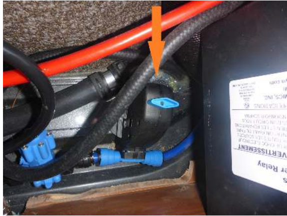
Alde frost control valve in operating position
