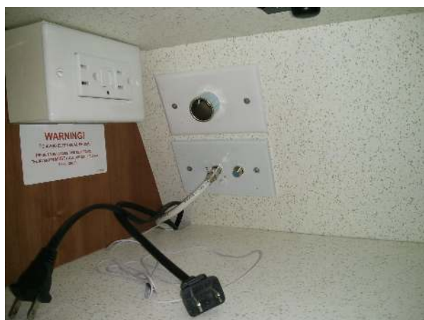
TV antenna and cable connections
