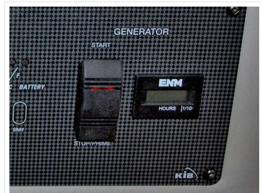
Propane generator control
