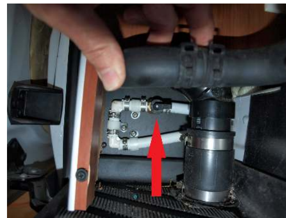
City water valve in open, along-the-line position
