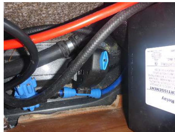
Frost protection valves turned to dump position - blue handle pointing toward water line, blue button at base is out
