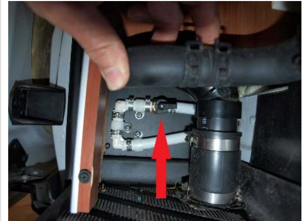
City water valve in open, along-the-line position
