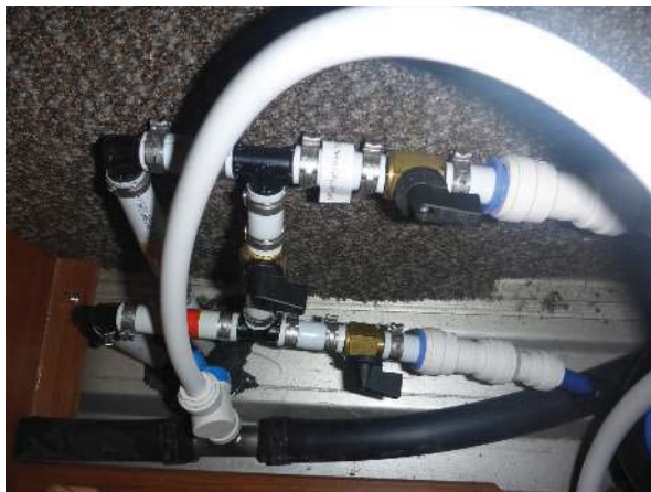
Bypass valves in normal position - all black handles horizontal
