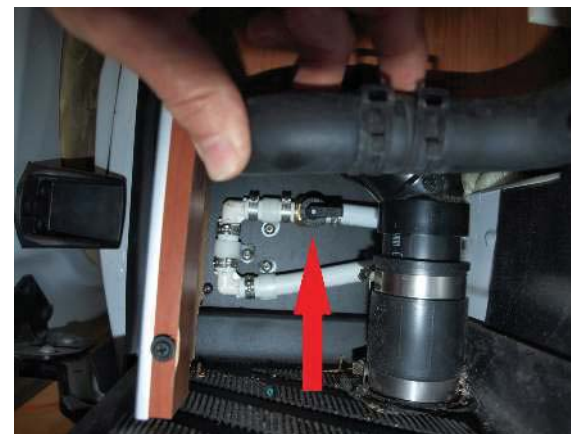
City water valve in open, along-the-line position
