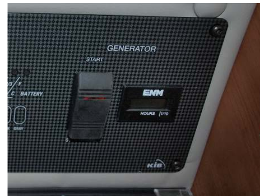
Generator switch and hour meter
