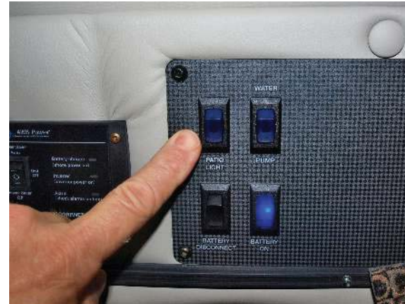
Patio light switch
