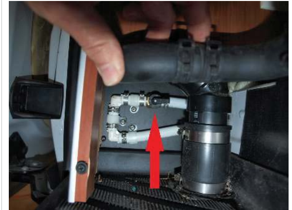
City water valve in open, along-the-line position
