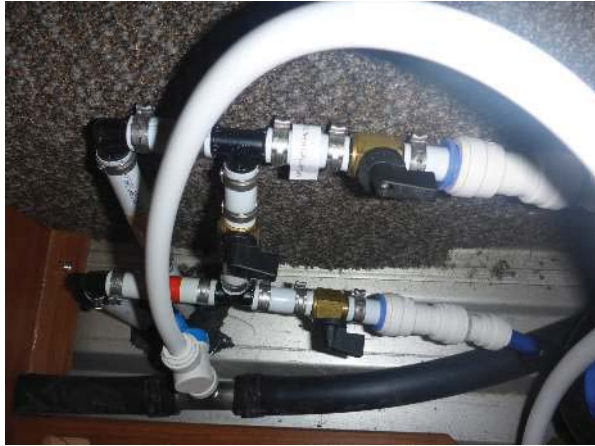
Alde bypass valves in normal operating position
