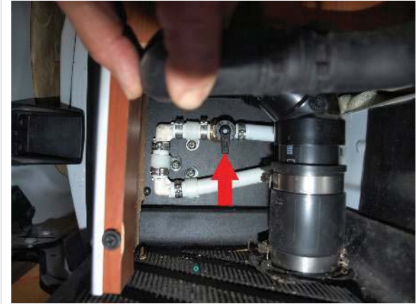
City water valve in closed, across-the-line position
