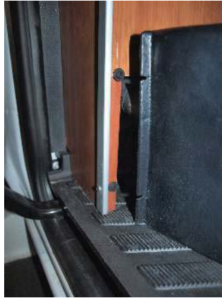
Screws holding plastic radiator cover on
