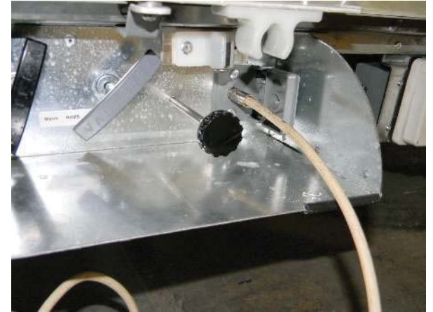
TV cable connected
