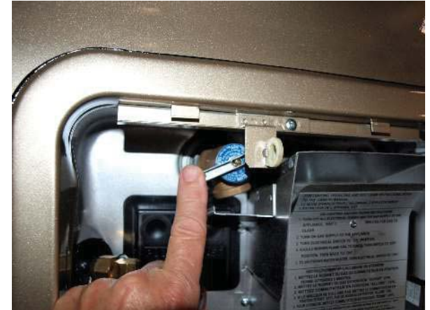
Water heater pressure relief valve
