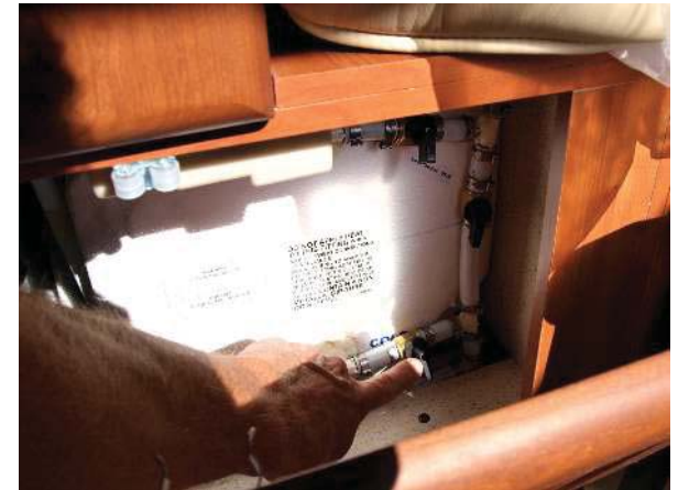
Water heater enclosure
