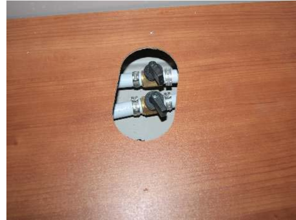
Valves for outside shower lines, shown closed
