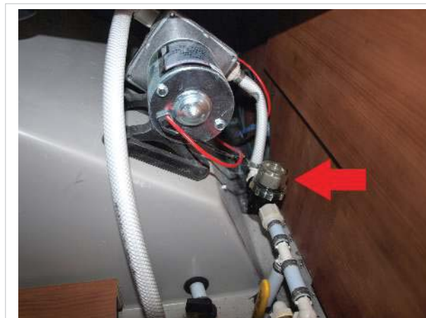
Water pump filter, inside water heater enclosure
