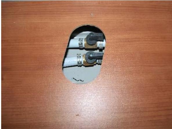
Valves for outside shower lines, shown open
