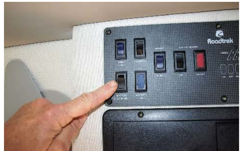
Battery disconnect switch
