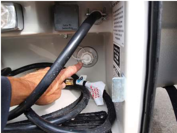
City water fill location
