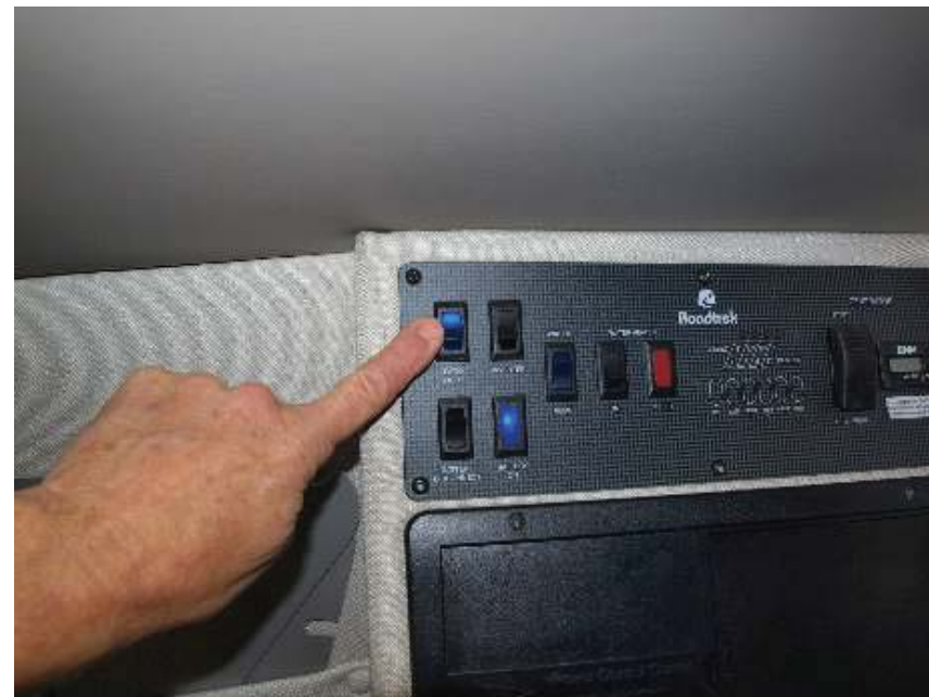
Patio light switch
