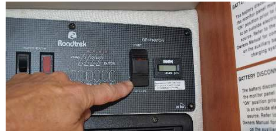
Generator switch, prime/off position
