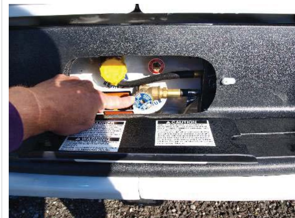
Propane tank main shutoff
