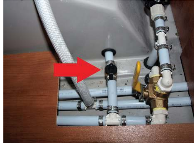
Tank isolator valve in open position
