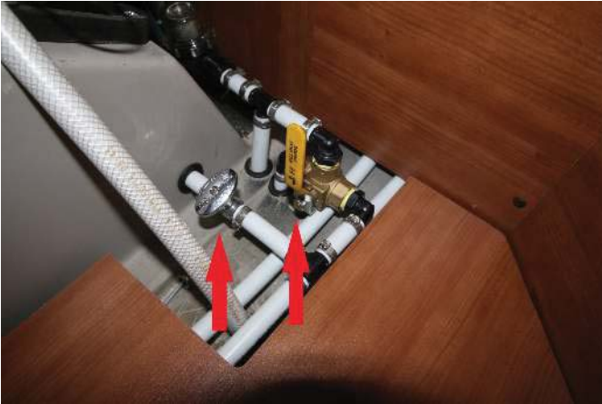
Tank selector valve on the left in closed or interior position. Tank selector valve on the right in interior tank position, with the colored plastic handle pointed up.
