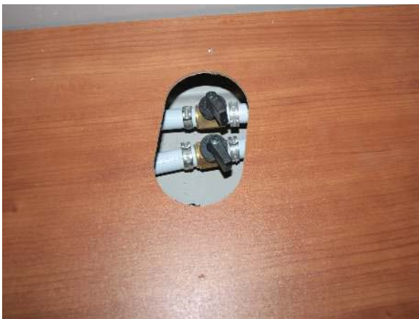
Outside shower valves, shown closed
