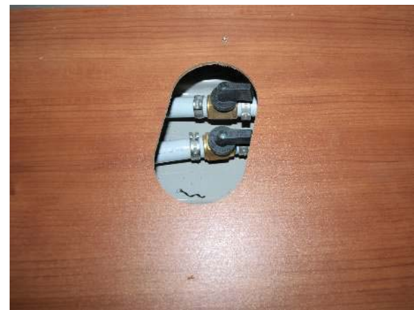
Outside shower valves, shown open
