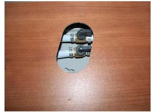
Outside shower valves, shown open
