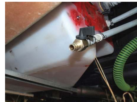
Exterior tank drain
