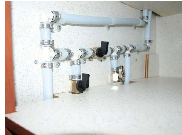
Water heater bypass valves in normal position - all handles vertical
