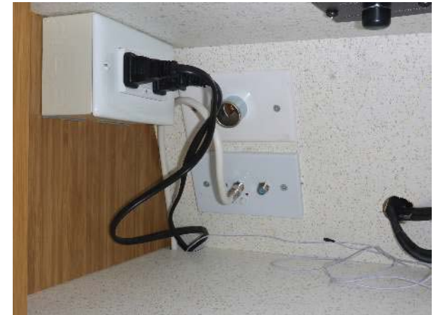
TV antenna switch and power injector
