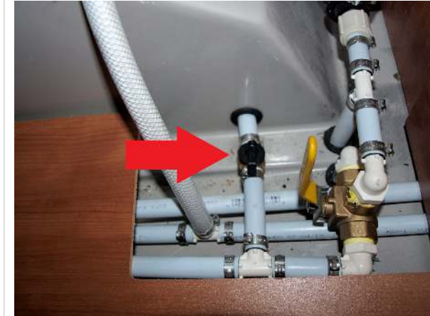
Tank isolator valve in open position
