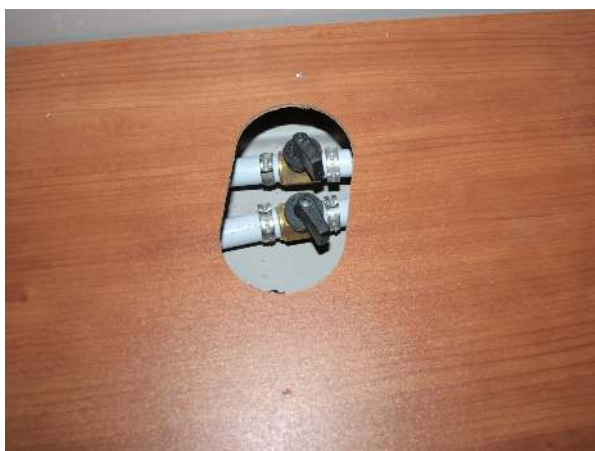
Outside shower valves, shown closed
