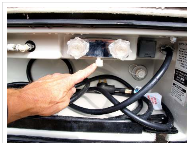
Outside shower connection
