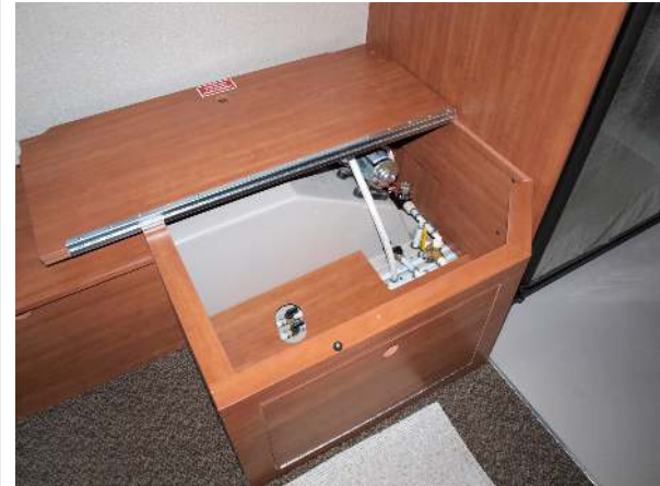
Water valves enclosure
