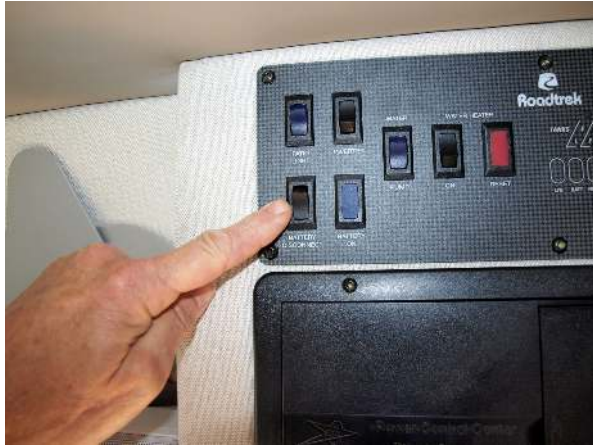
Battery disconnect switch
