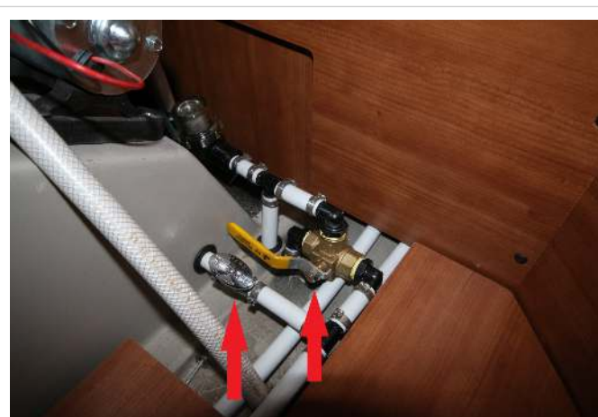
Tank selector lever in the exterior (horizontal) position
