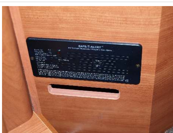
Propane and CO alarm
