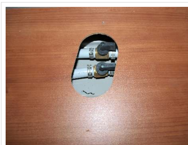
Outside shower valves, shown open
