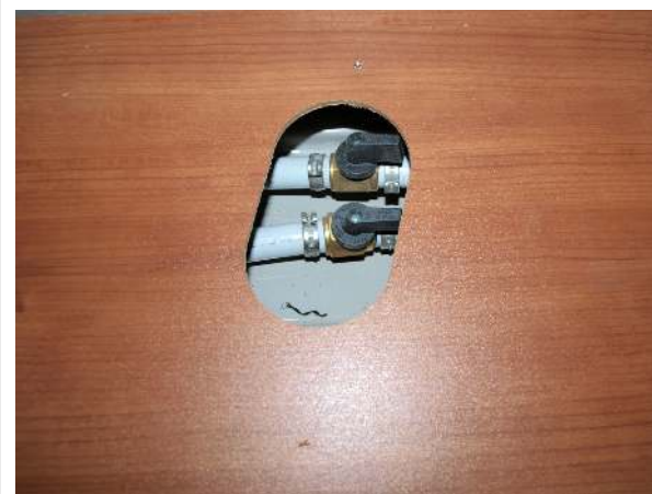
Outside shower valves, shown open
