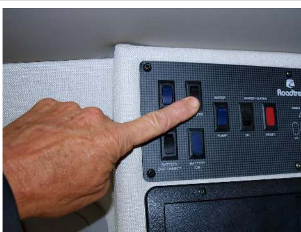
Inverter switch with standard 750 watt inverter
