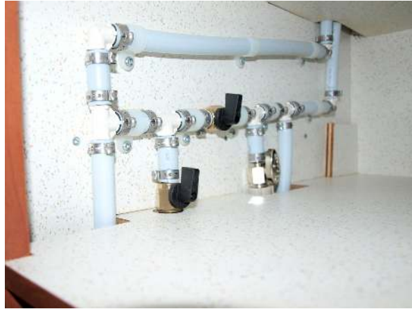
Water heater bypass valves in the unwinterized, normal position
