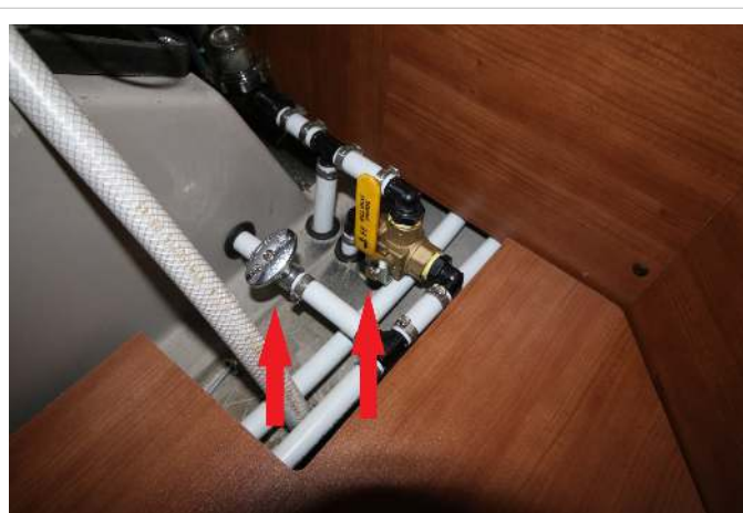
Tank selector valve on the left in closed or interior position. Tank selector valve on the right in interior tank position, with the colored plastic handle pointed up.
