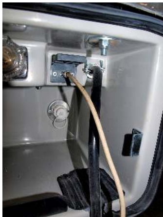
TV cable connected
