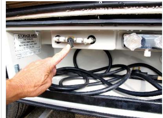
City water valve in closed position
