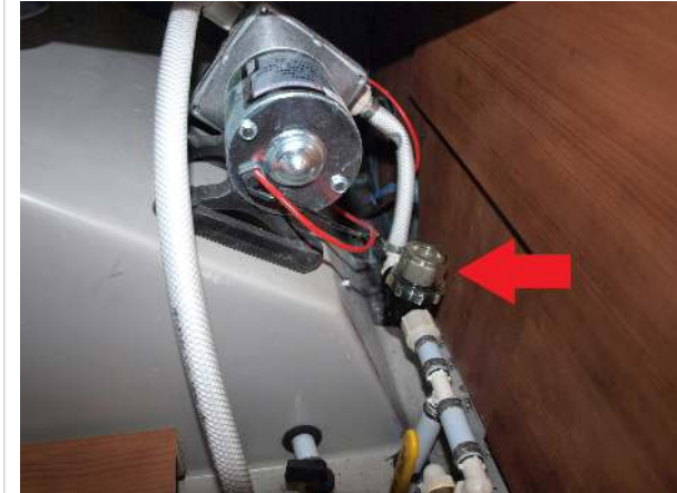
Water pump filter, inside water heater enclosure
