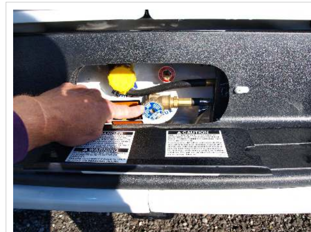
Propane tank main shutoff
