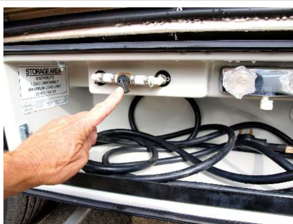
City water connection valve, shown closed
