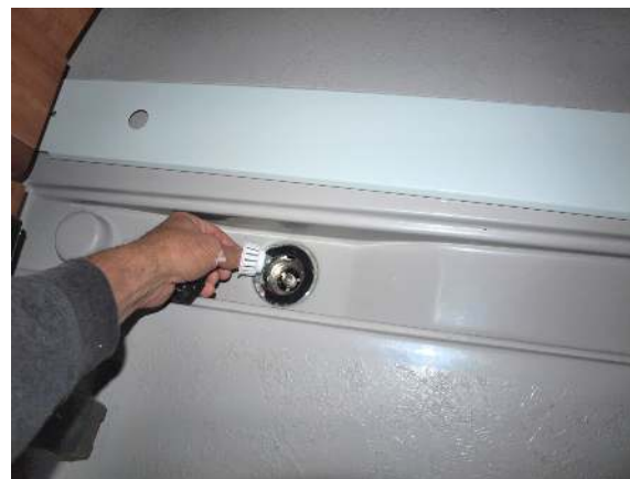
Aisle shower drain
