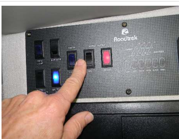
Water heater switch and red indicator light
