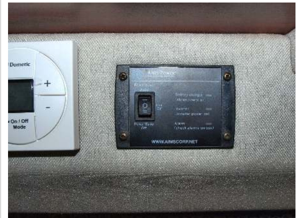
Inverter switch for big inverter
