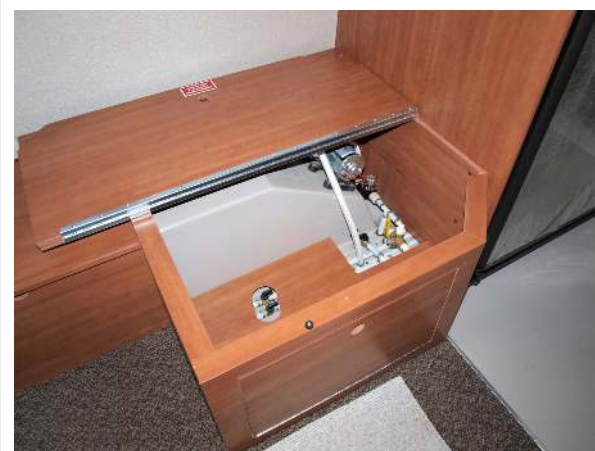
Lid raised to expose valves and water pump
