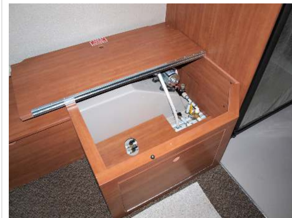
Water valves enclosure
