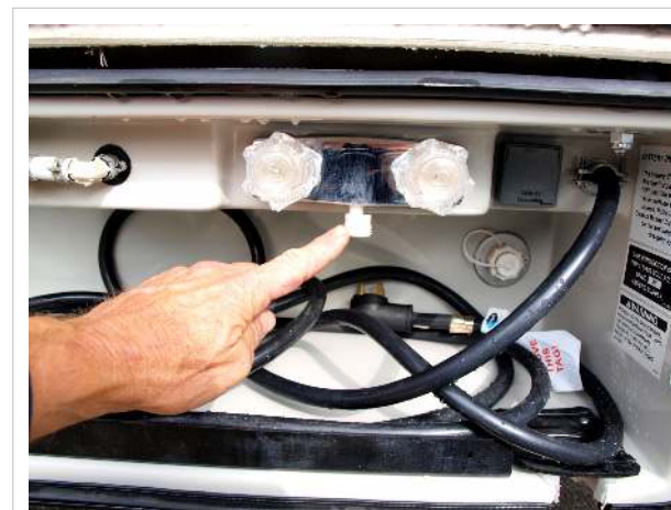
Outside shower connection
