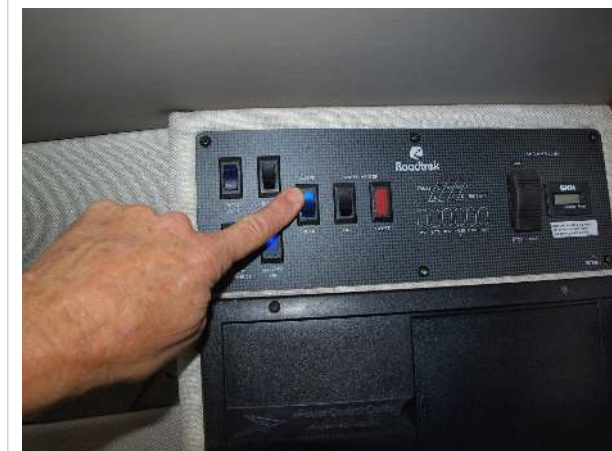
Water pump switch
