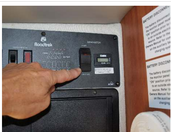
Generator switch, prime/off position
