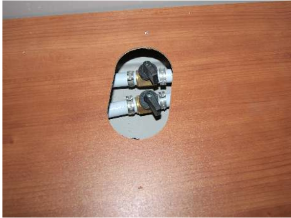
Outside shower valves, shown closed
