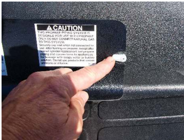
Propane access cover
