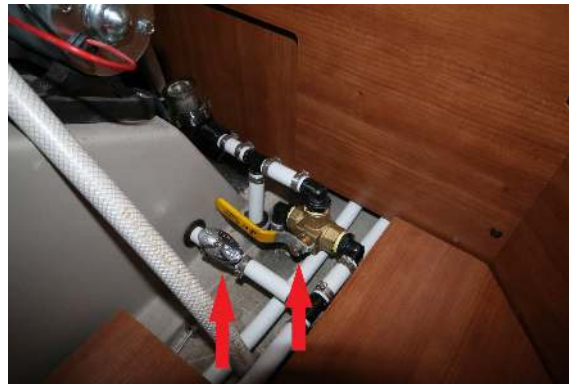
Tank isolation valve on the left in open or connected position; tank selection valve on the right in exterior tank position
