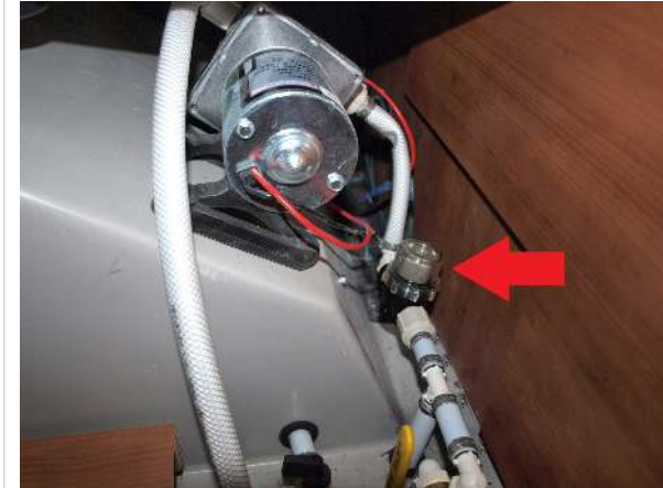
Water pump filter, inside water heater enclosure
