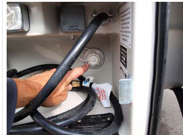
City water connection
