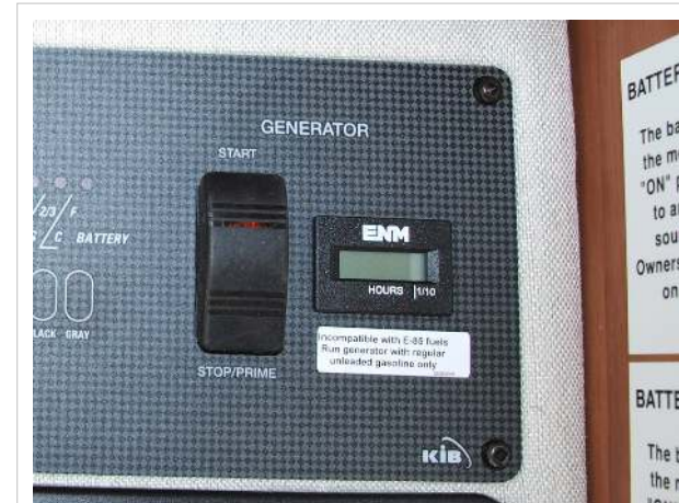
Generator switch and hour meter
