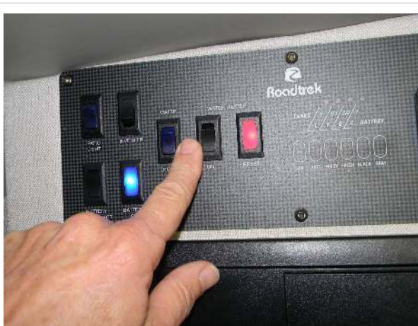
Water heater switch and red indicator light
