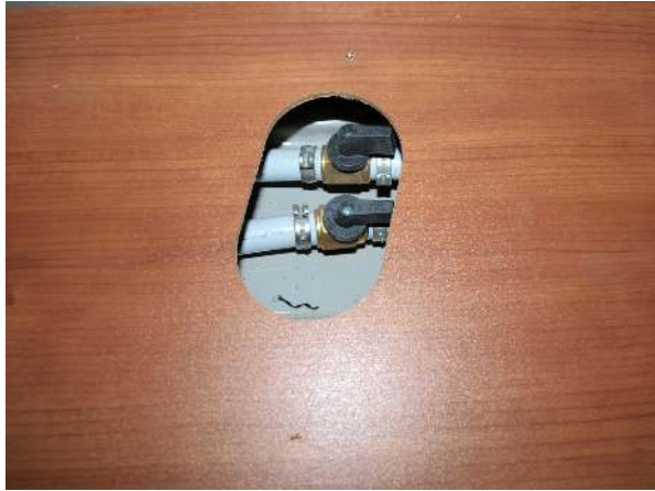
Valves for outside shower lines, shown open
