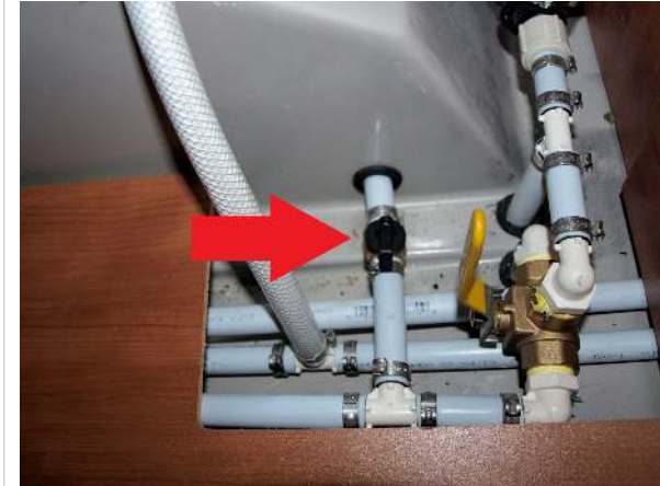
Tank isolator valve in open position
