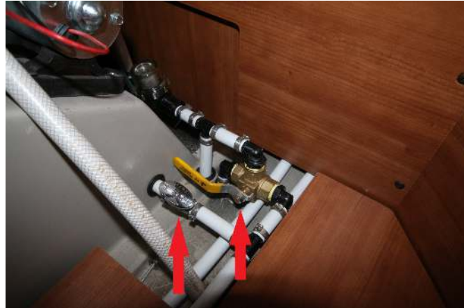
Tank selector valve in exterior tank position
