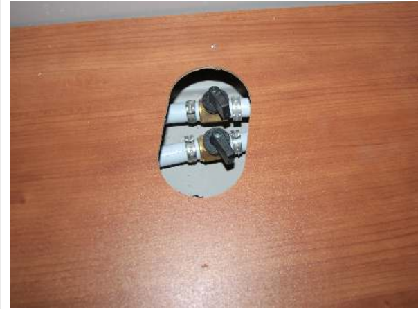
Valves for outside shower lines, shown closed
