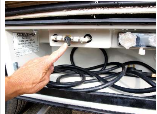
City water valve in closed position
