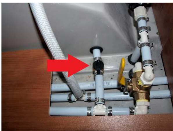
Location of the tank isolator valve shown in the open (i.e. tanks connected) position; note valve is in-line with pipe
