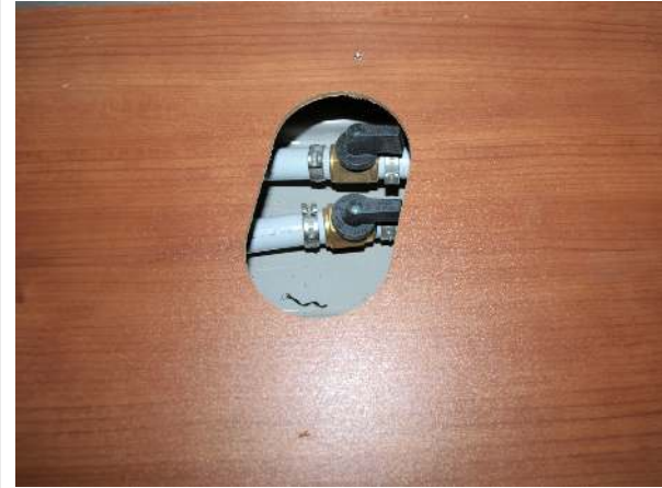
Outside shower valves, shown open
