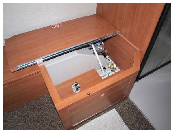
Lid raised to expose valves and water pump
