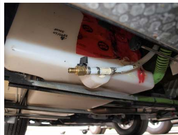
Freshwater tank drain valve, shown closed
