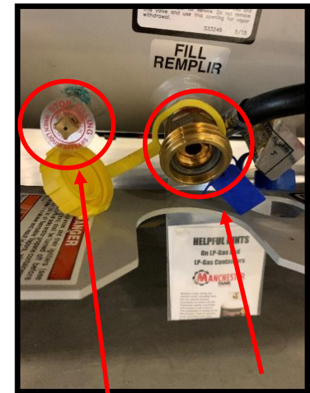
Propane bleed valve and propane fill valve
