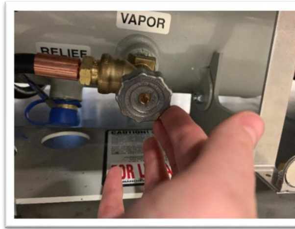
Propane tank main shutoff valve
