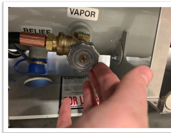
Propane tank main shutoff valve
