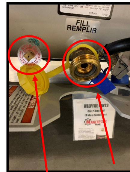
Propane bleed valve and propane fill valve
