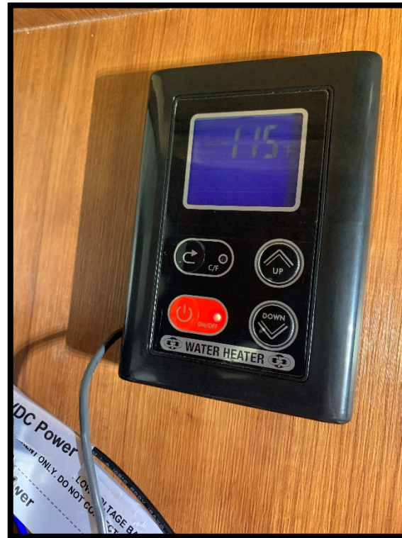
26.3 Water heater control panel
