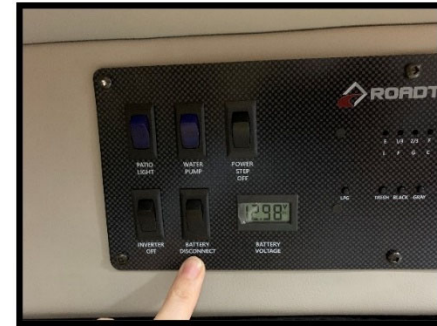
Battery Disconnect Switch 43.3
