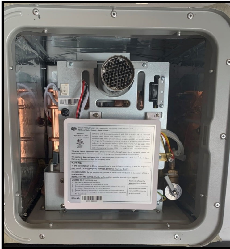
26.2 Girard water heater
