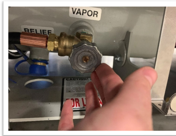
Propane tank main shutoff valve
