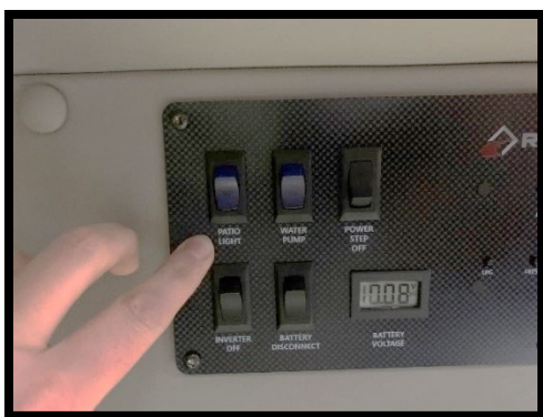
44.1 Patio Light Switch
