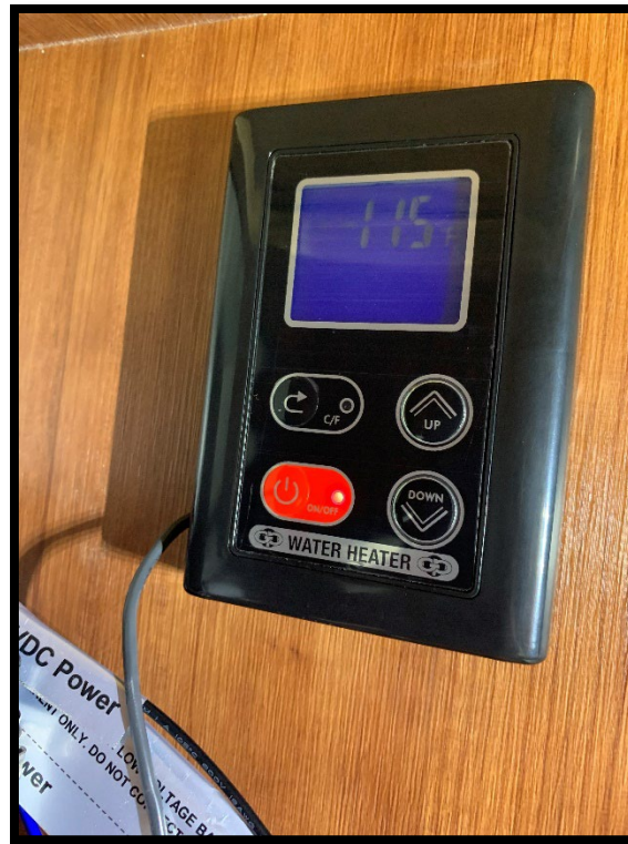
26.3 Water heater control panel
