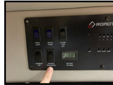
Battery Disconnect Switch 43.3
