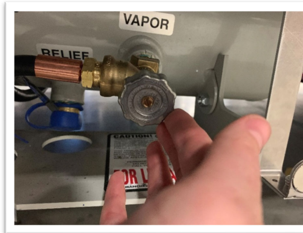
Propane tank main shutoff valve
