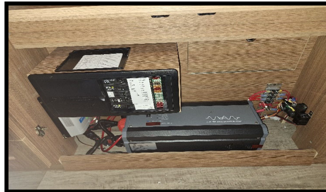
Breaker and fuse panel in the electrical cabinet
