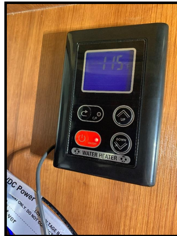
26.3 Water heater control panel
