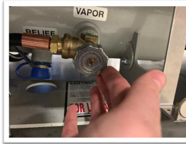
Propane tank main shutoff valve
