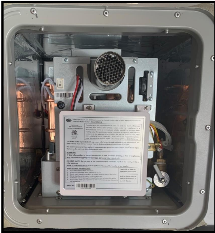
28.2 Girard water heater
