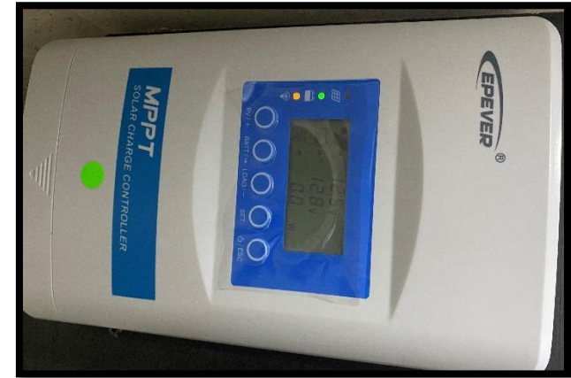
Solar charge controller
