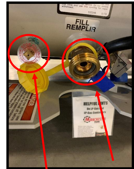
Propane bleed valve and propane fill valve
