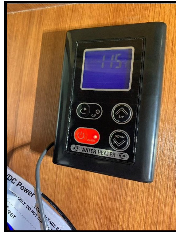
26.3 Water heater control panel
