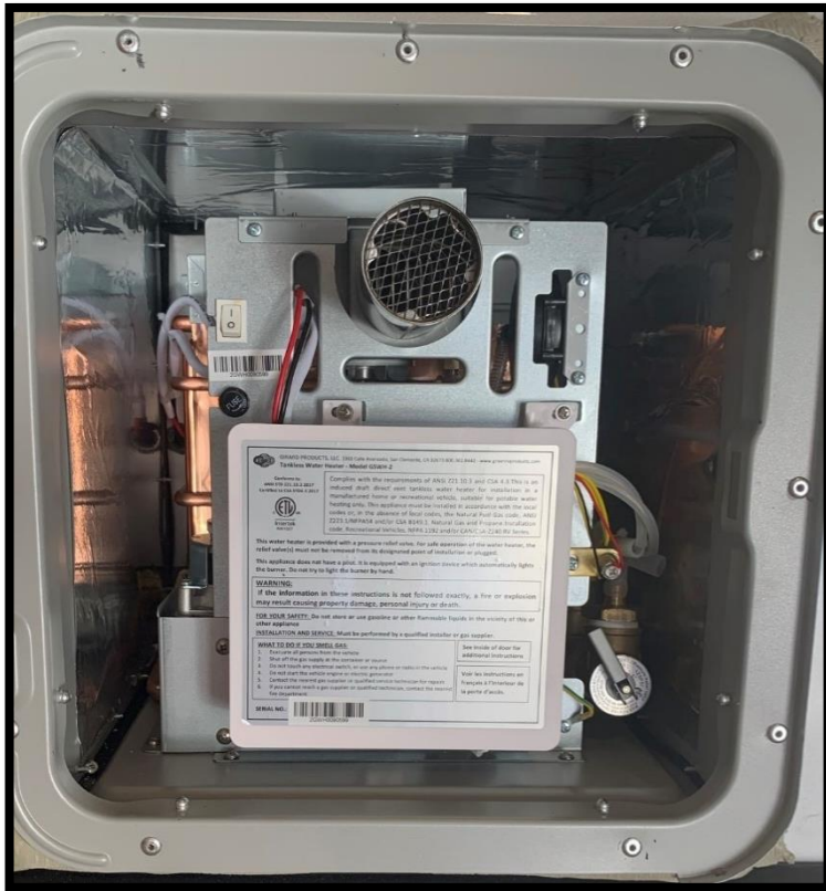
26.2 Girard water heater
