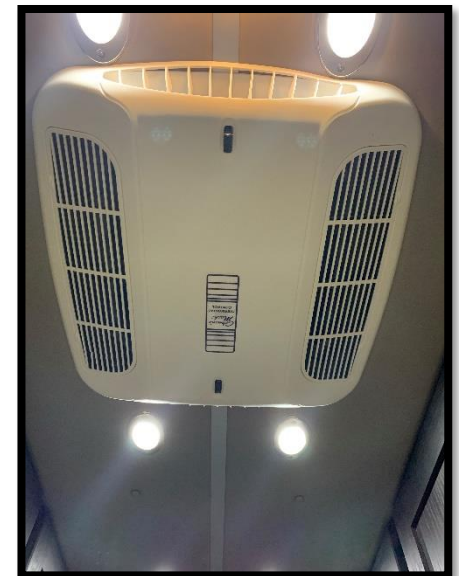
35.3 Roof-mount air conditioner
