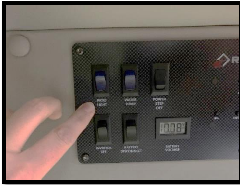
44.1 Patio Light Switch
