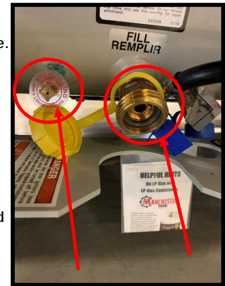
Propane bleed valve and propane fill valve
