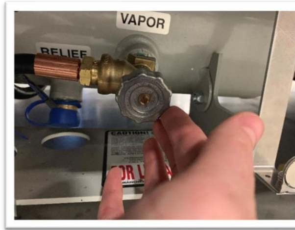
Propane tank main shutoff valve
