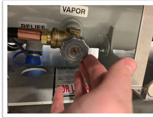
Propane tank main shutoff valve
