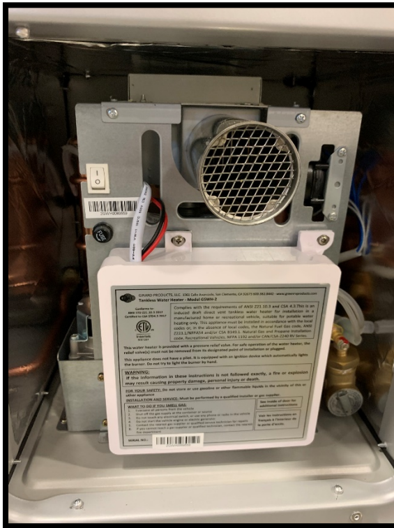
Picture 29.2 Girard water heater
