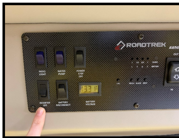
Picture 40.2 Inverter switch
