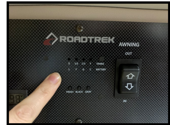
Picture 43.1 Tank Indicators
