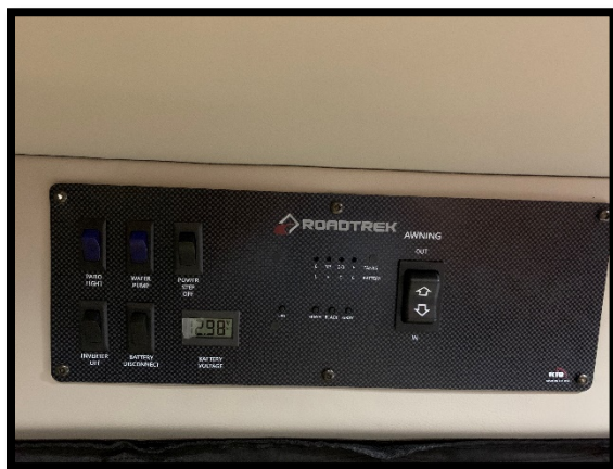
Picture 40.1 Monitor Panel
