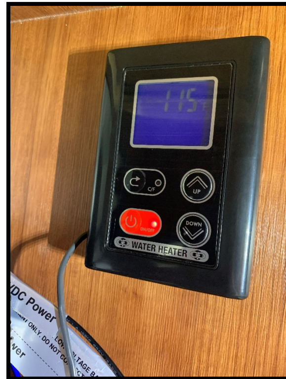
Picture 29.3 Water heater control panel
