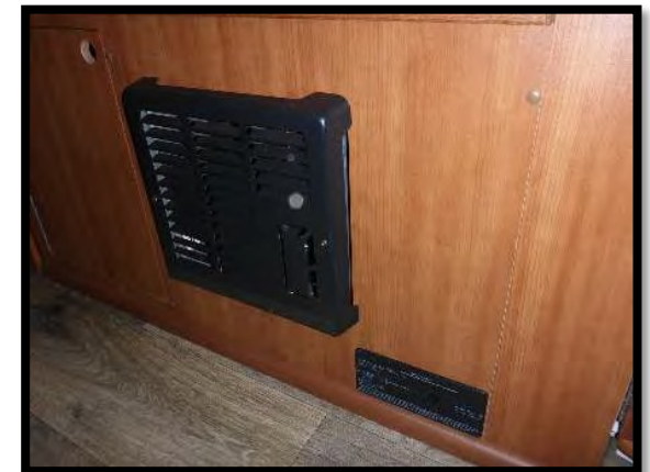
Picture 36.2 Propane Furnace
