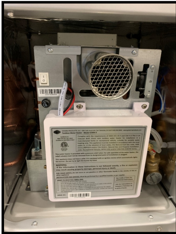
Picture 29.2 Girard water heater
