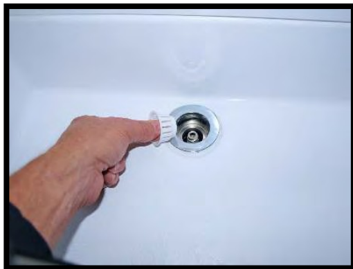
Picture 26.2 Shower drain
