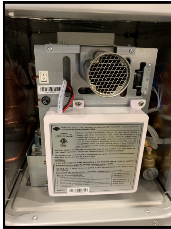
Picture 29.2 Girard water heater
