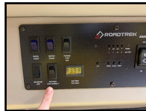
Picture 40.3 Battery disconnect switch
