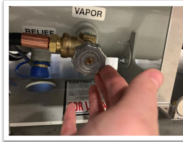
Propane tank main shutoff valve
