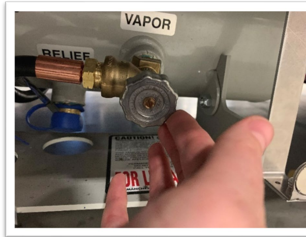
Propane tank main shutoff valve
