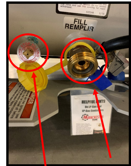
Propane bleed valve and propane fill valve
