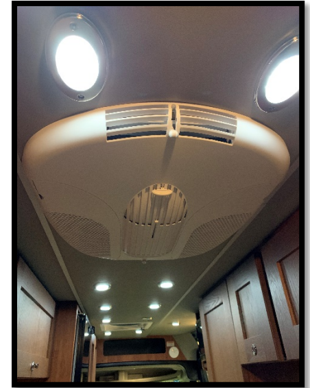
Picture 36.3 Roof-mount air conditioner
