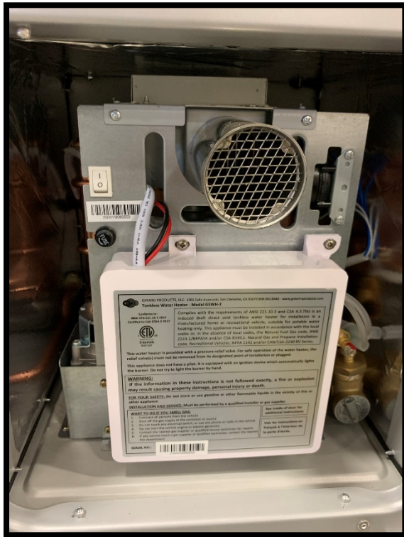
Picture 29.2 Girard water heater
