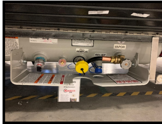
Picture 36.5 Propane tank
