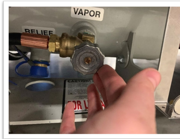
Propane tank main shutoff valve
