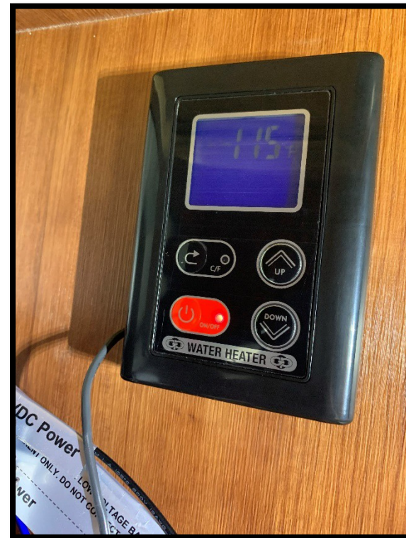
Picture 29.3 Water heater control panel
