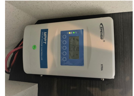
Picture 38.1 Solar charge controller
