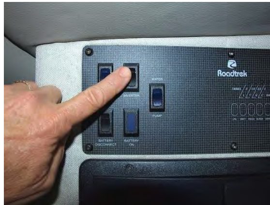
Picture 40.2 Inverter switch
