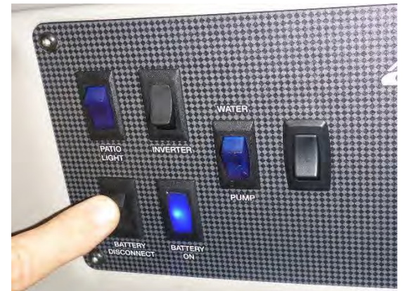
Picture 40.3 Battery disconnect switch
