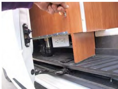
The freshwater fill valve is behind this access panel to the left of the side door opening
