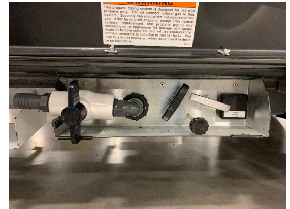
Wastewater hose, dump valves, pump cleaning knob, and CATV connection
