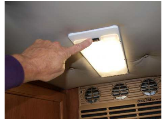
Picture 15.3 Fluorescent light
