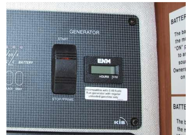
Generator switch and hour meter
