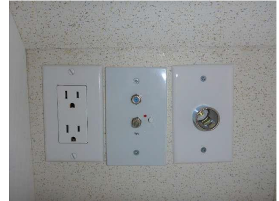
TV Antenna and Cable connections
