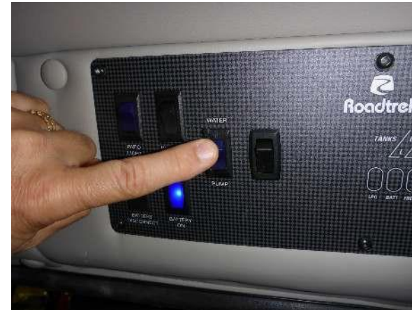
Water pump switch
