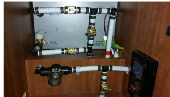
Water heater thermostat, filter and drain valves
