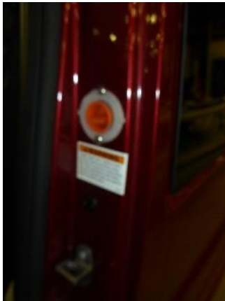
Fresh water tank fill
