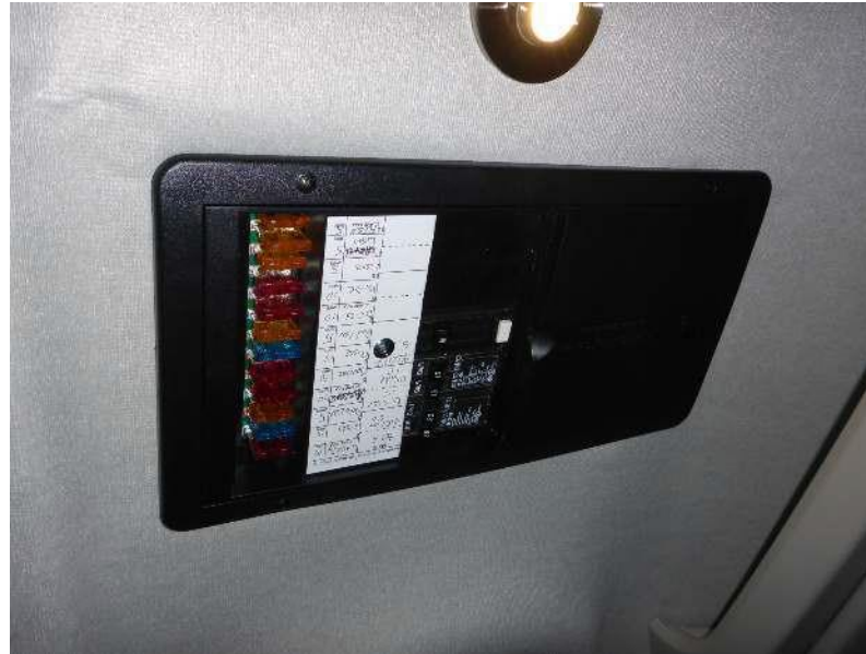
Breaker and fuse access
