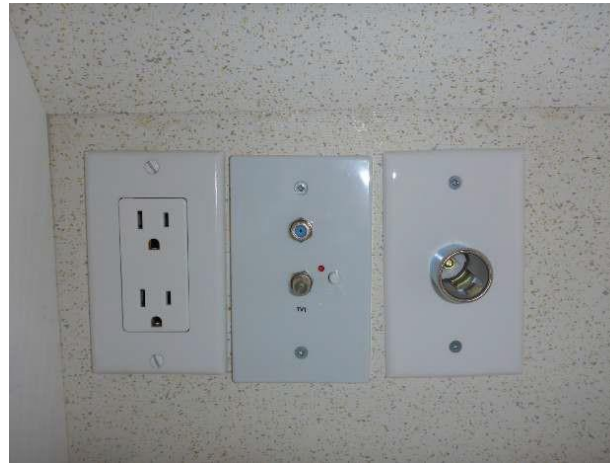
TV Antenna and Cable connections
