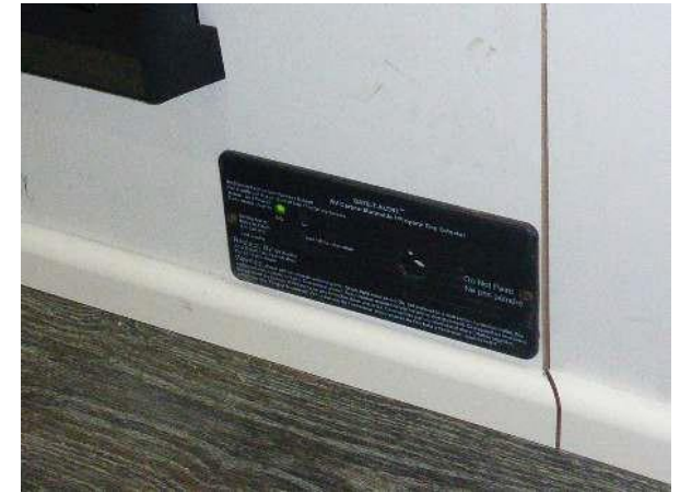
Propane and Carbon Monoxide alarm
