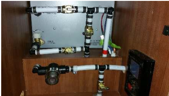
Water heater thermostat, filter and drain valves
