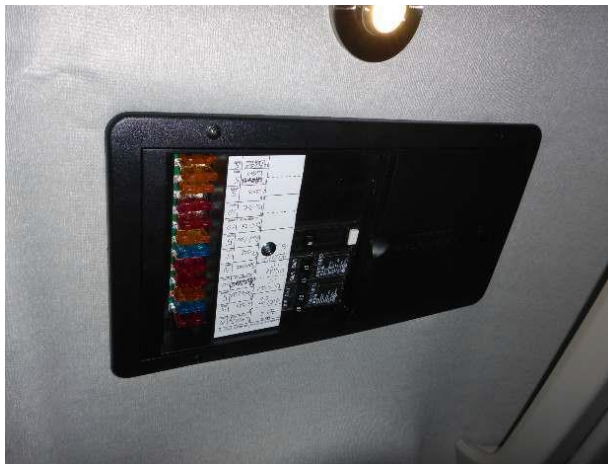
Breaker and fuse access
