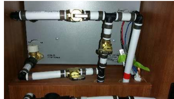
Tankless water heater inside cabinet – all valves are in normal operating position
