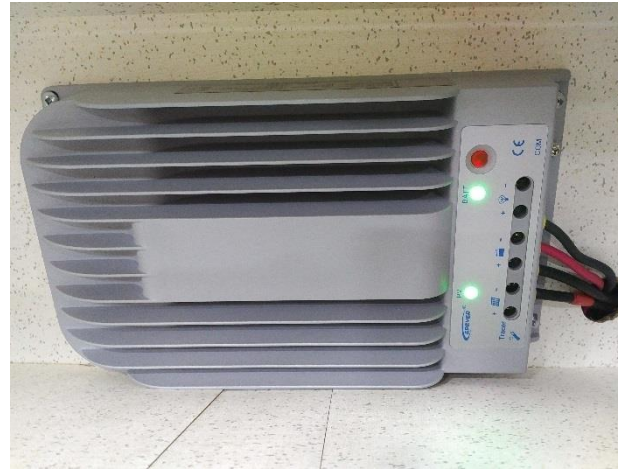
Solar controller in cabinet above galley
