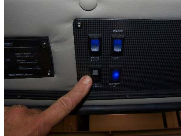
Battery disconnect switch
