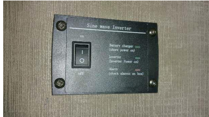
Inverter Control Panel
