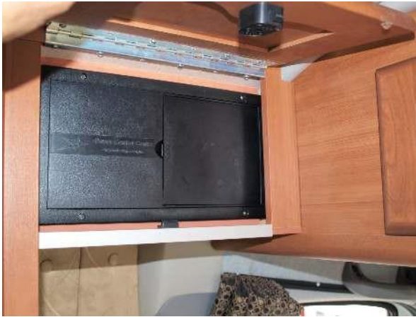
Agile power distribution panel location
