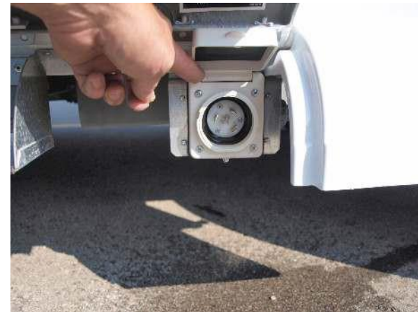
Shore power connection
