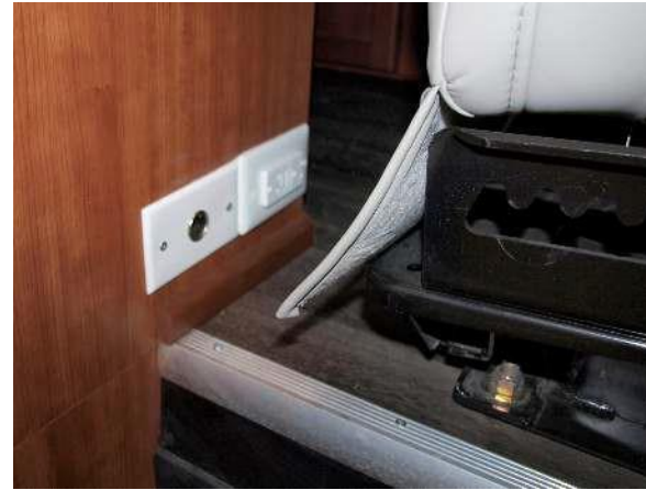
GFCI plug behind rear captain's seat
