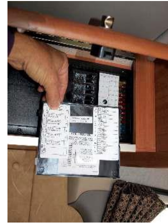
Agile AC breakers and 12 volt fuses
