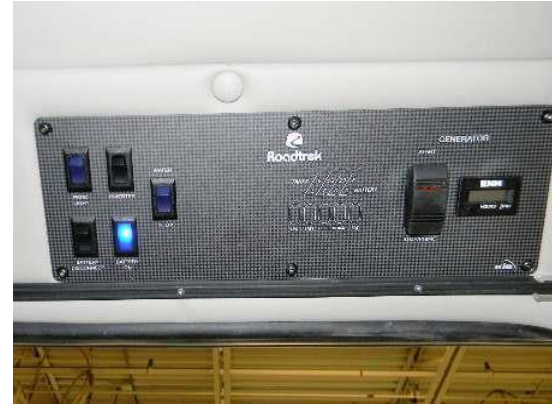
Monitor panel for unit's propane generator
