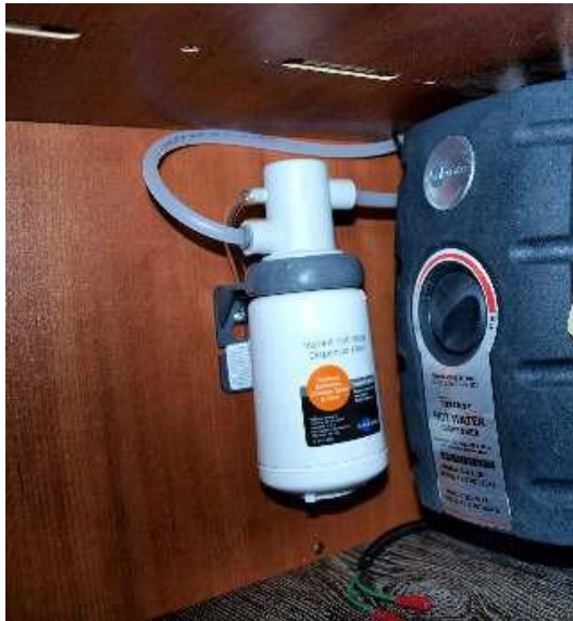
On-demand hot water system filter
