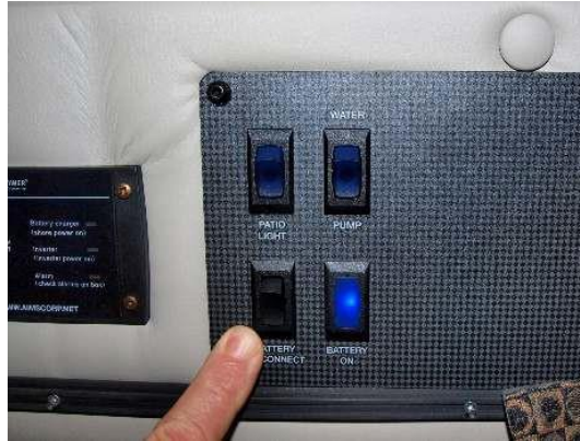
Battery disconnect switch
