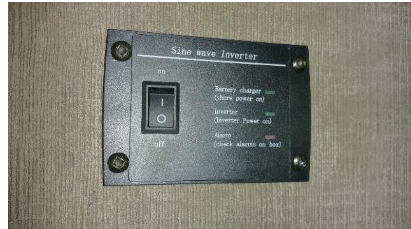
Inverter Control Panel
