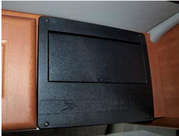
120AC breaker panel showing breakers and stickers
