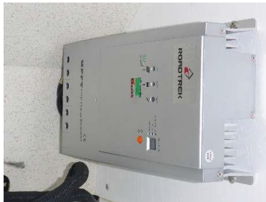
Solar controller in cabinet above galley
