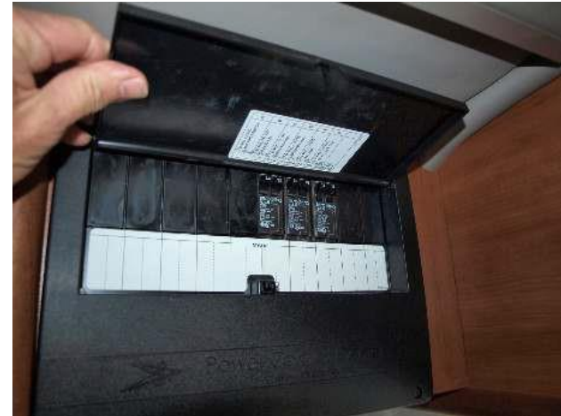
120AC breaker panel showing breakers and stickers
