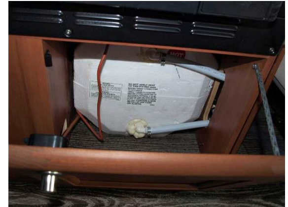
Water heater below microwave oven
