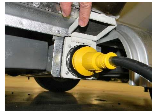
Attached shore power cord
