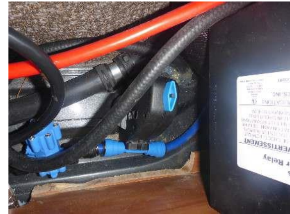
Frost control valve in tripped position
