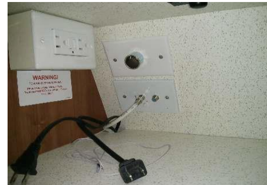
TV antenna and cable connections
