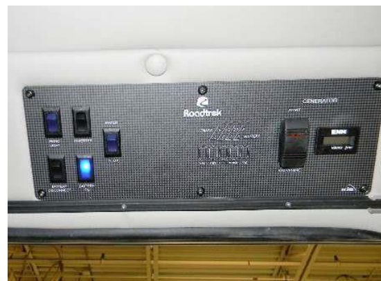
Monitor panel for units propane generator
