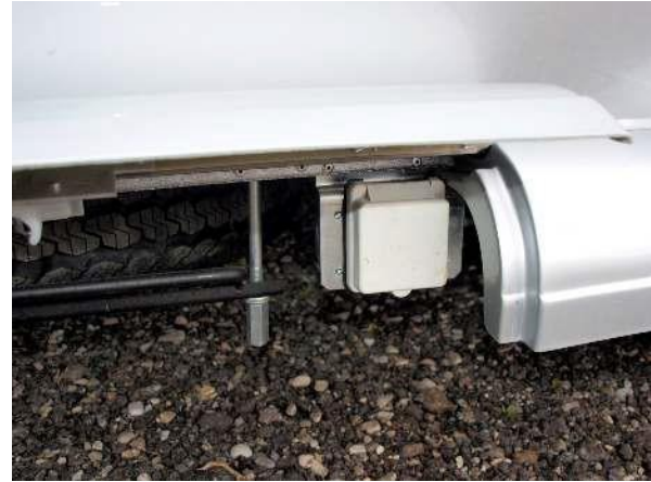
Shore Power connection point
