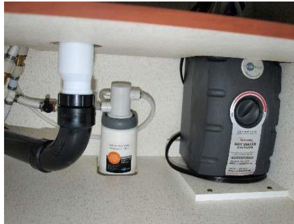
On demand hot water system filter
