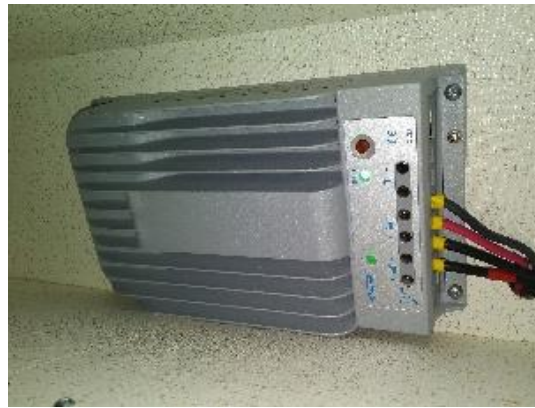
Solar controller in cabinet above galley
