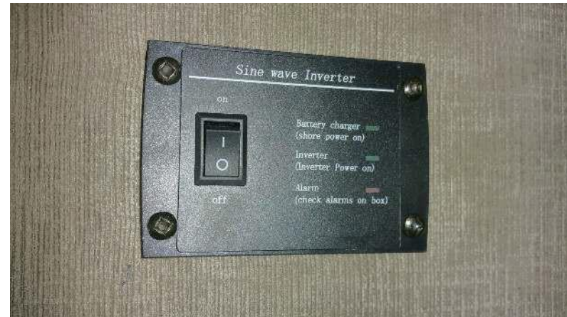
Inverter Control Panel
