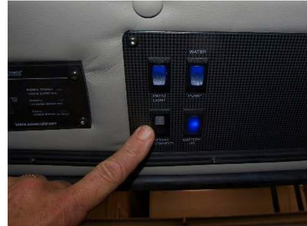
Battery disconnect switch
