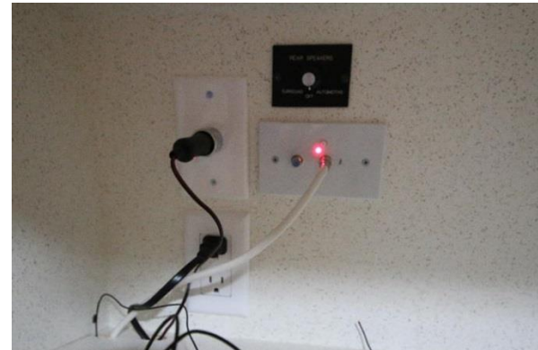
TV antenna and cable connections
