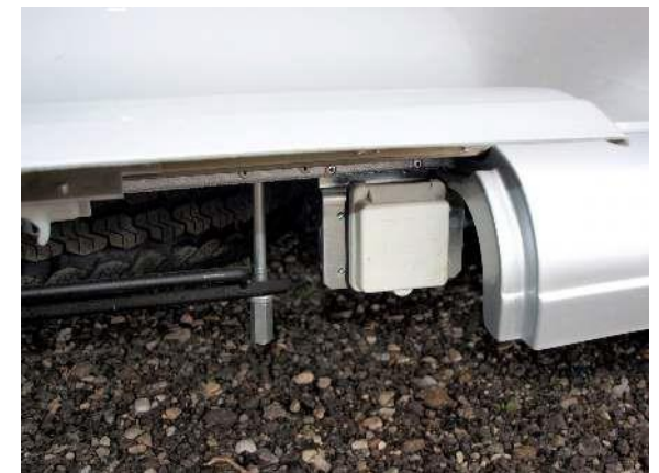
Shore power connection
