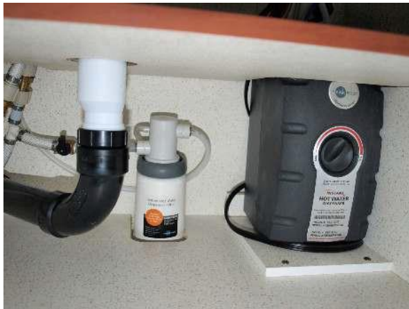
On-demand hot water system filter
