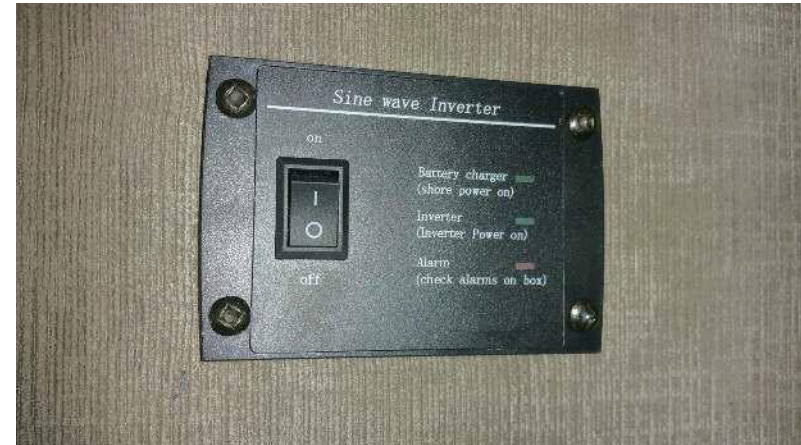
Inverter Control Panel
