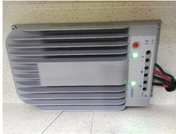
Solar controller in cabinet above galley
