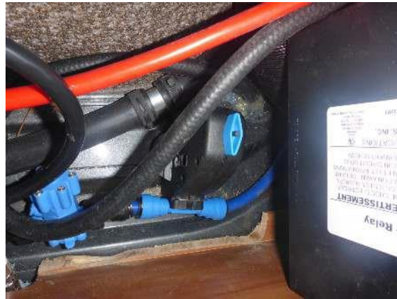
Front control valve in tripped position
