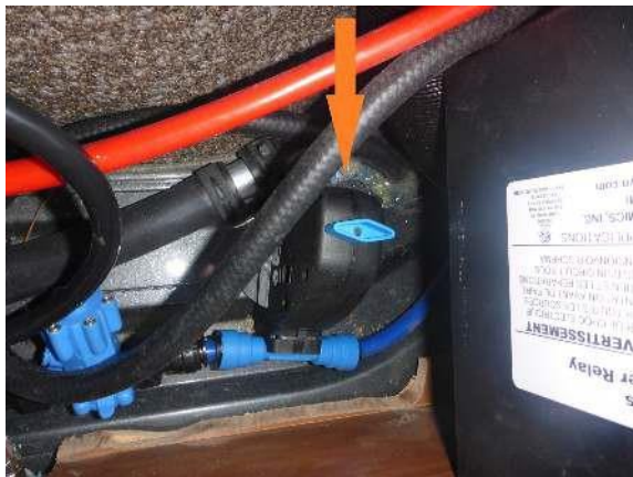
Alde frost control valve in operating position
