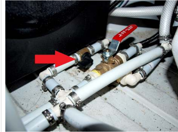
Tank isolator valve in open position
