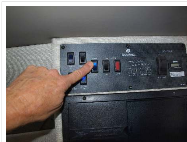
Water pump switch
