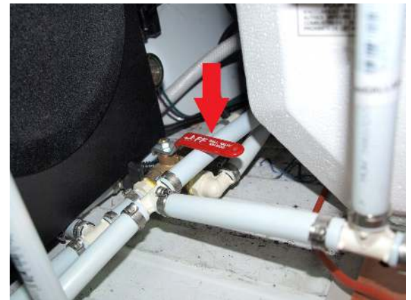
Tank selector valve in interior tank position
