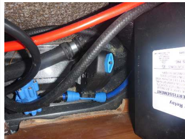
Resetting the tripped valve
