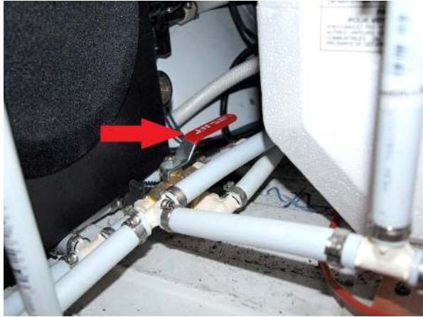
Tank selector valve in exterior tank position
