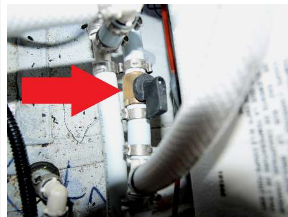
Cold water shutoff valve, shown open
