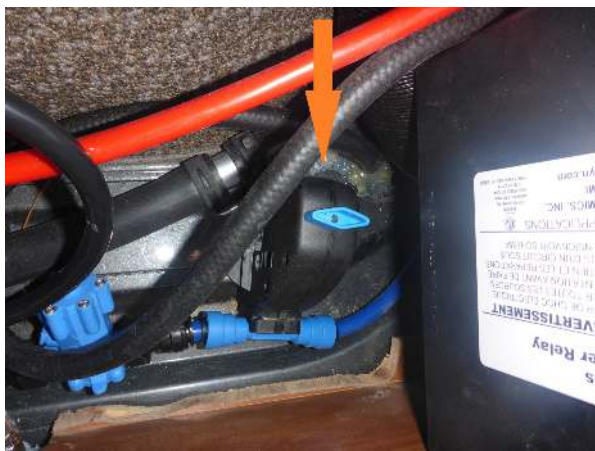
Alde frost control valve in operating position
