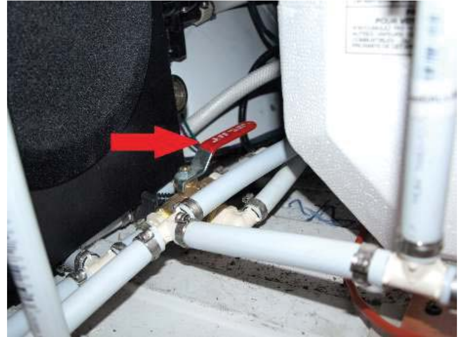
Tank selector lever in the exterior position
