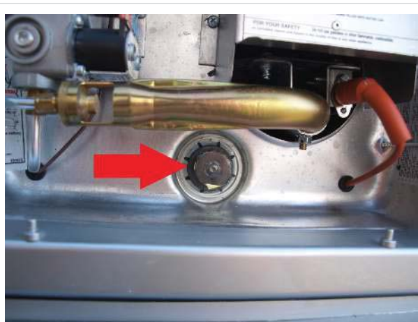
Water Heater Anode
