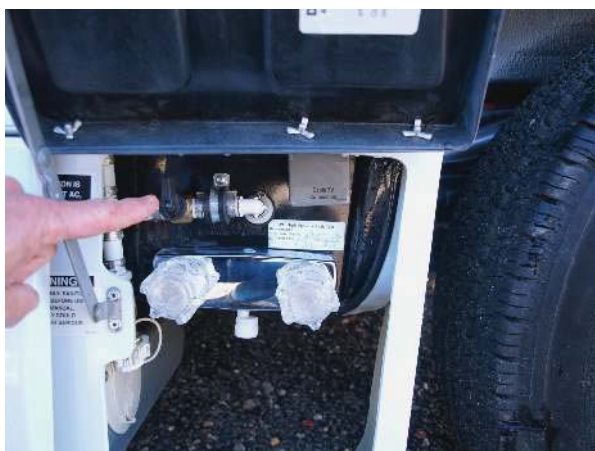
City water connection valve
