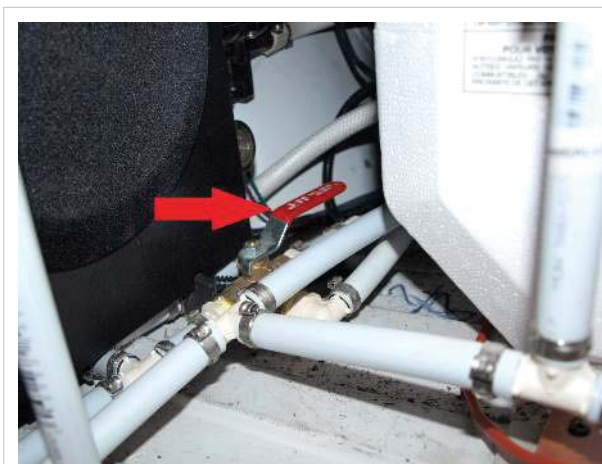
Tank selector lever in the exterior position
