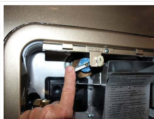
Water heater pressure relief valve
