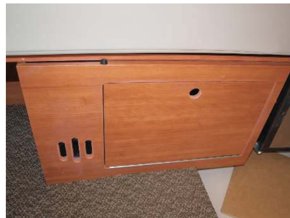
Water heater cabinet
