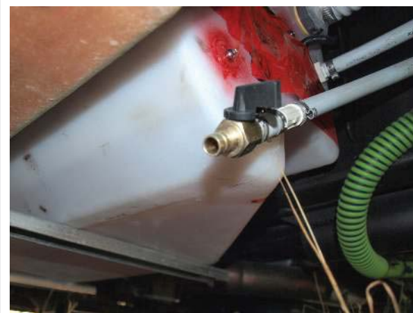
Freshwater tank drain valve
