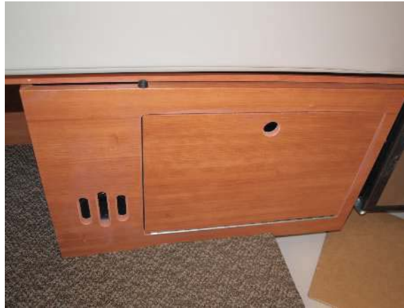
Water heater enclosure
