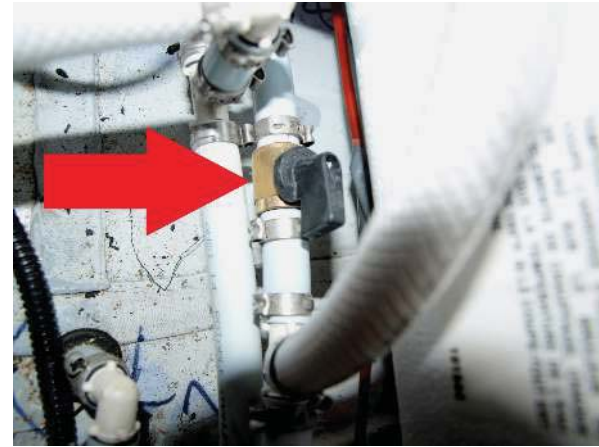
Cold water shutoff valve, shown open
