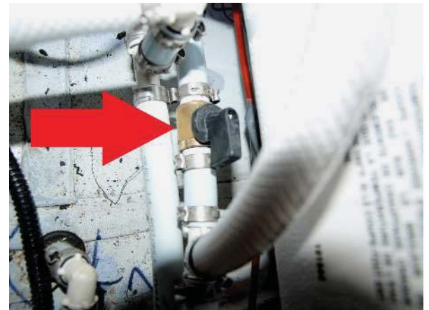
Cold water shutoff valve, shown open
